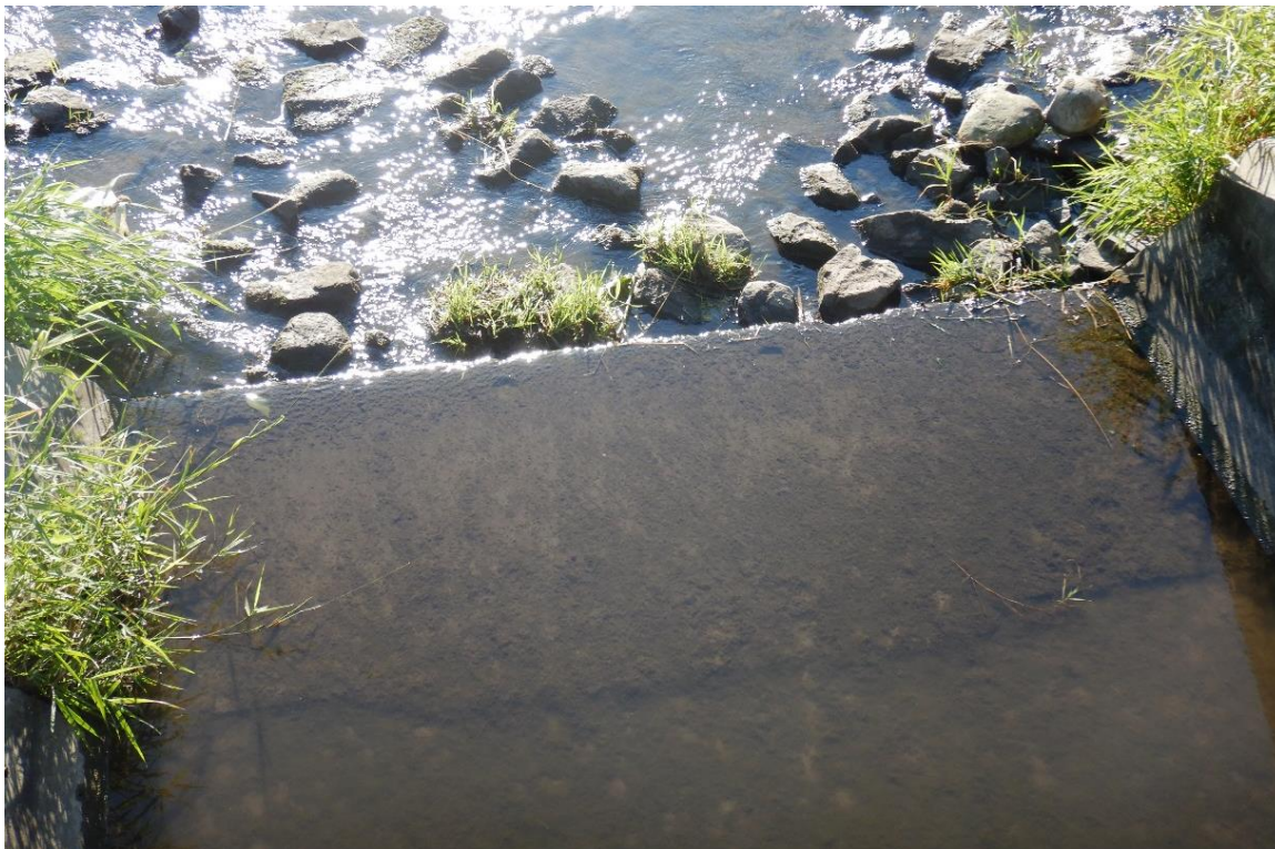
Figure 20. Perched culvert at site 17MN170 (8/29/2019)
