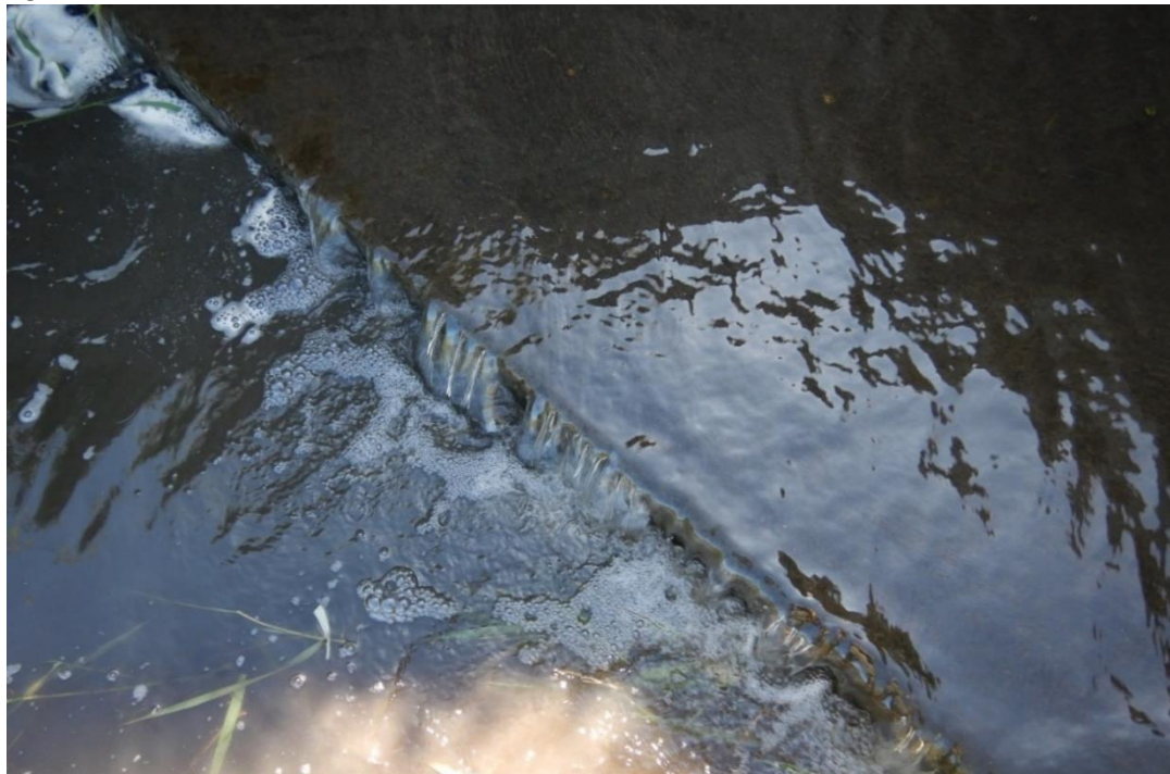
Figure 40. Perched culvert at site 17MN176
