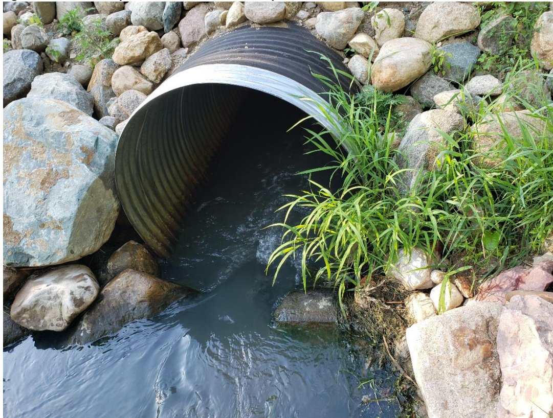
Figure 34. Incorrect slope on culvert on Dutch Charley Creek
