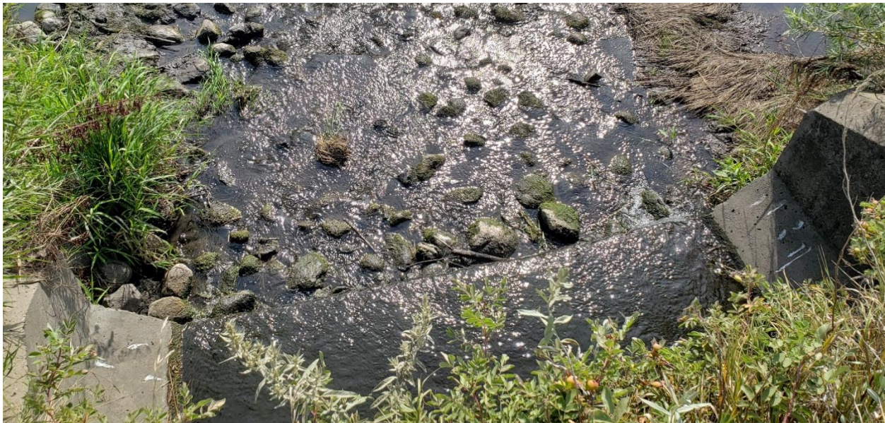
Figure 56. Perched culvert at site 91MN065 (8/22/19)
