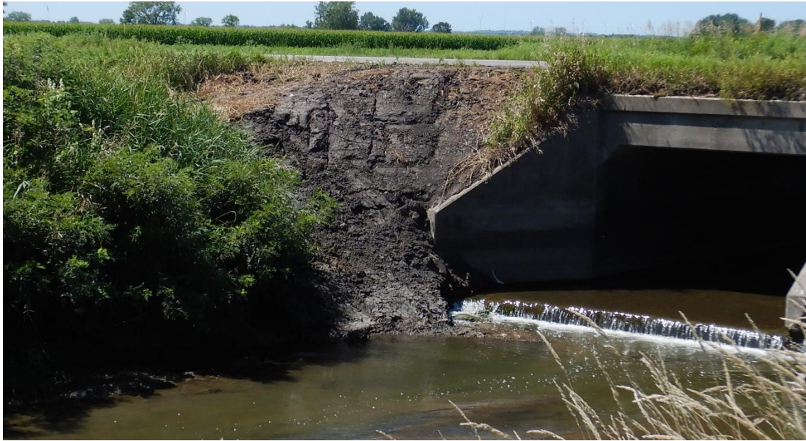
Figure 19. Perched culvert at site 17MN171 (8/8/2019)
