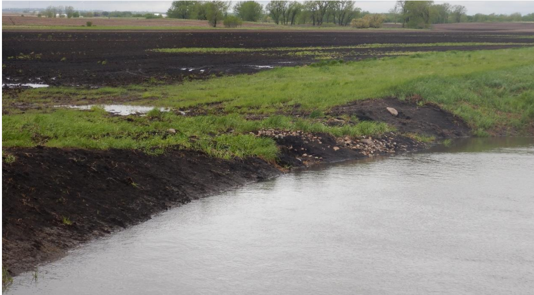
Figure 15. Eroding bank along site 17MN165 (5/22/2019)
