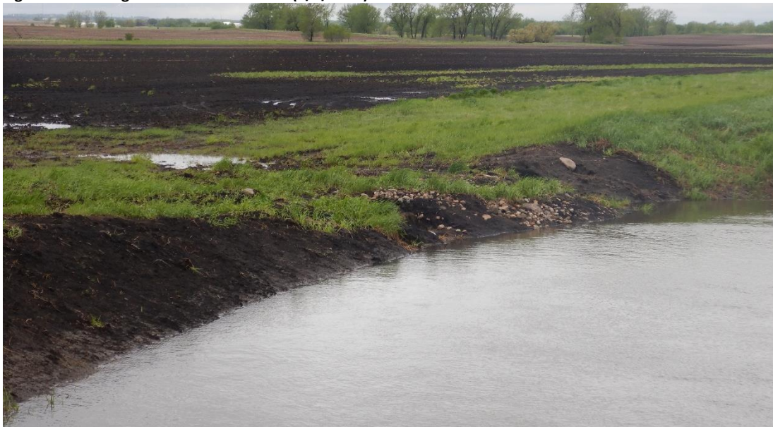
Figure 16. Eroding bank at site 17MN171 (8/8/2019)
