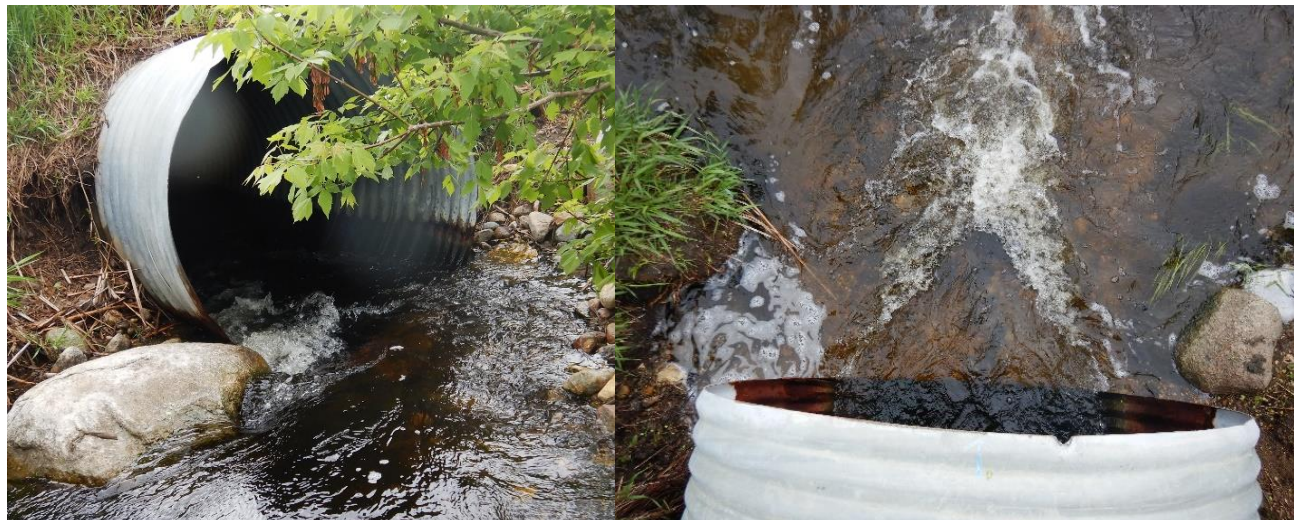
Figure 21. Perched culvert at site 17MN164 (5/22/2019)
