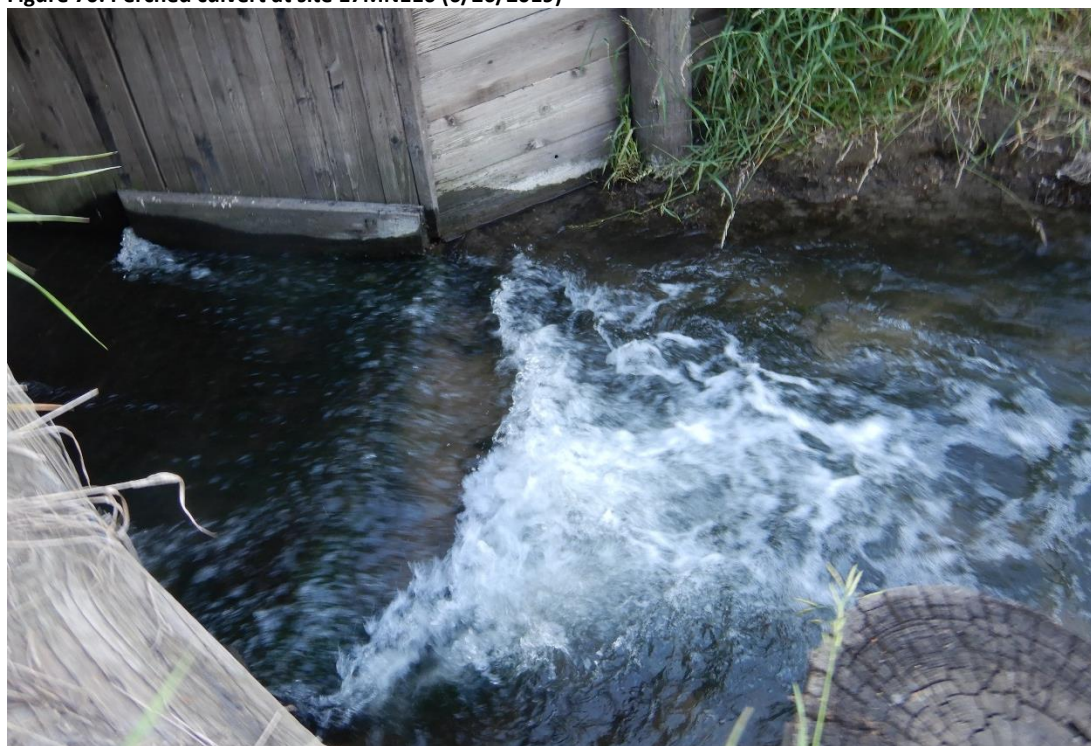
Figure 70. Perched culvert at site 17MN116 (6/26/2019)
