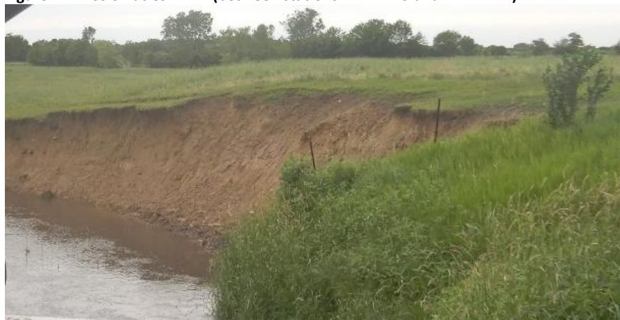
Figure 44. Erosion at CSAH 11 (between stations 17MN129 and 17MN127)
