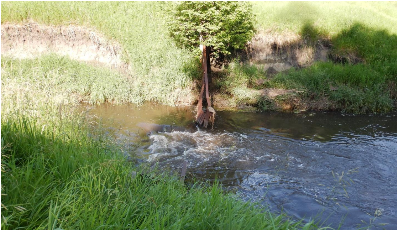
Figure 74. Barrier at 17MN107 (6/26/2019)
