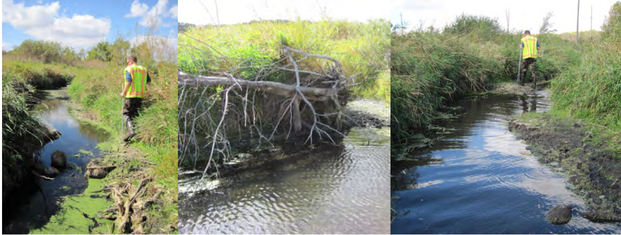
Figure 628-8: Station 09MN007 (Note soft soil stream bottom and bank erosion).
