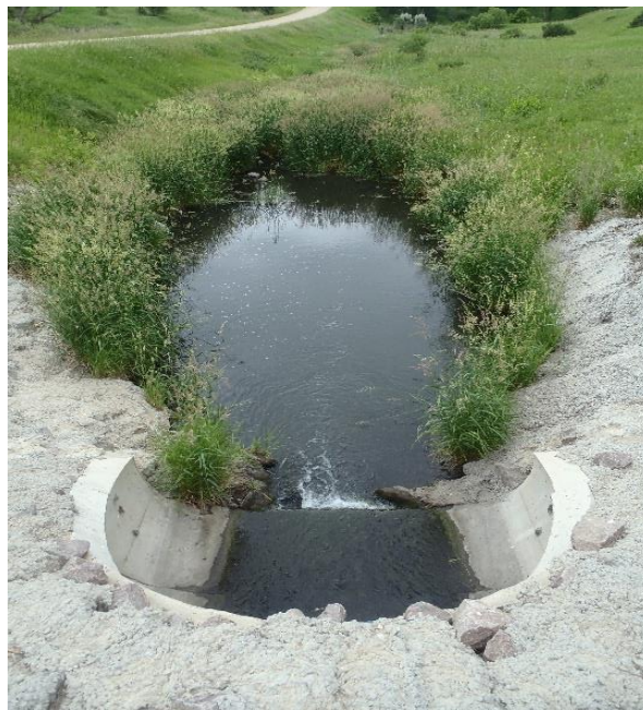
Figure 12. Photo of culvert, a possible fish barrier, just upstream of Bio site 15MN002
