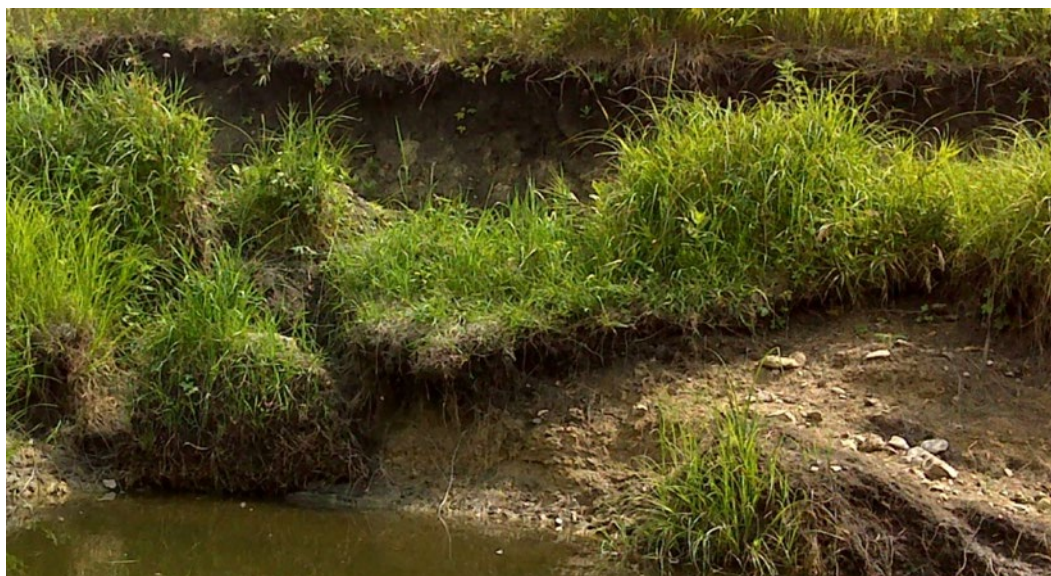
Figure 46. Eroding bank along the South Fork Crow River (August 7, 2013)
