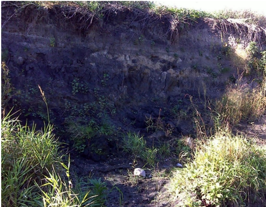
Figure 114. Erosion at station 12UM006 (October 9, 2013)
