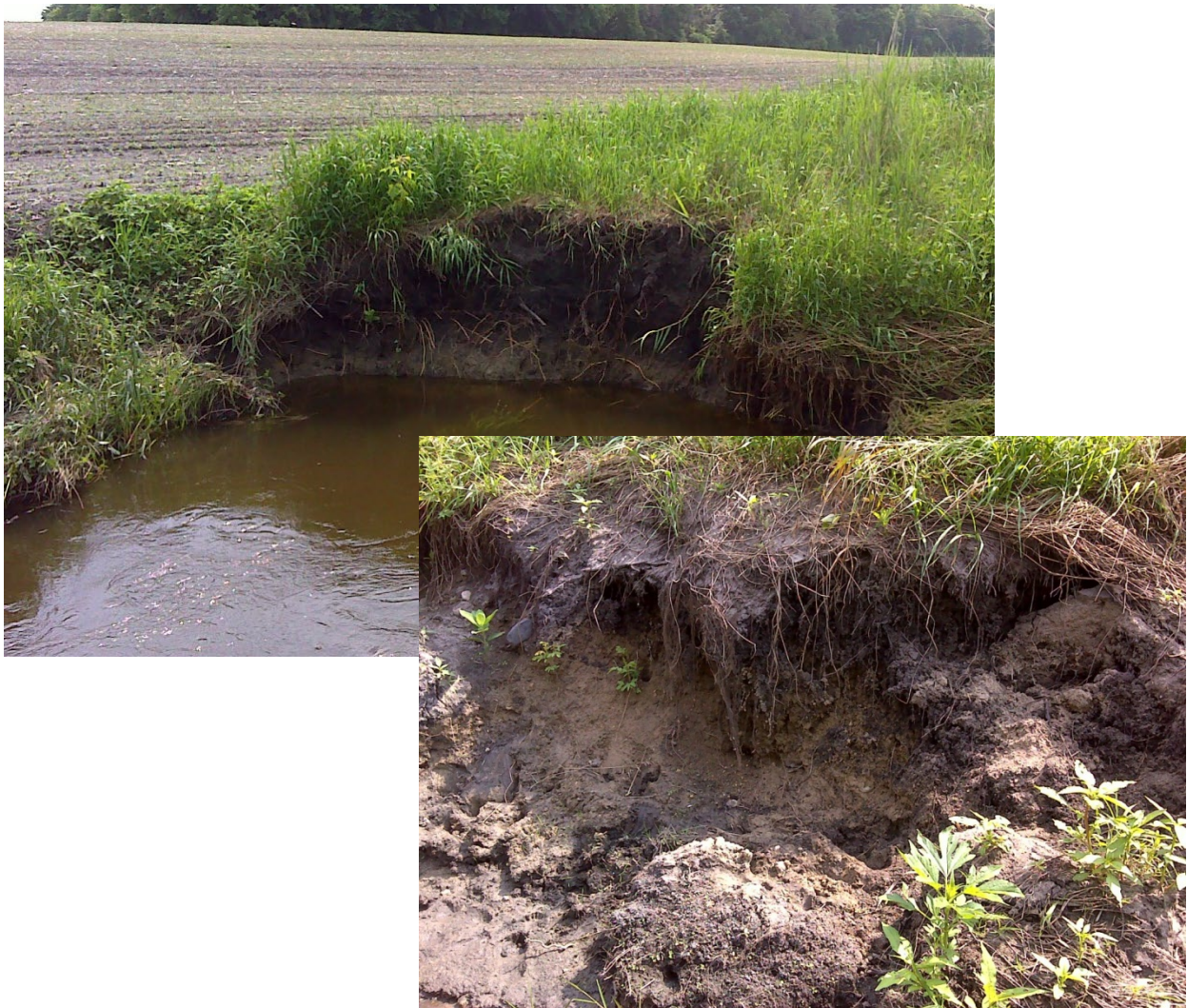
Figure 127. Bank erosion at 12UM022 (top) and 12UM024 (bottom)
