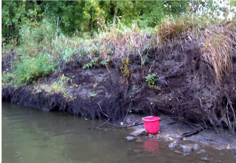
Figure 68. Eroding bank at station 14UM001 (October 3, 2013)
