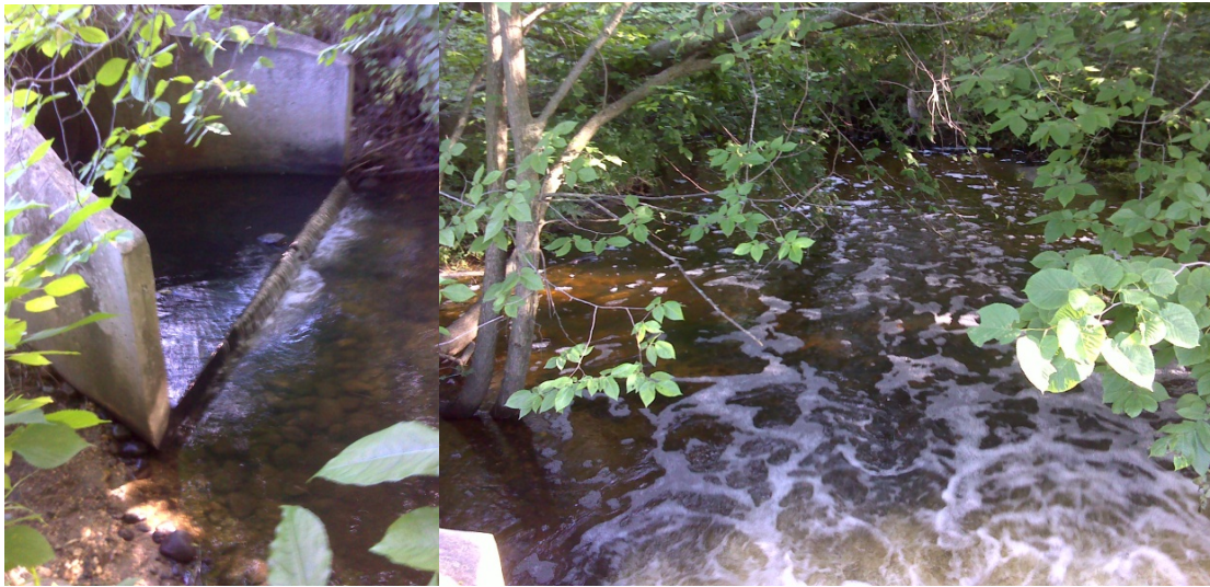
Figure 37: Unnamed Creek culvert outlet on County Road 14 on July 2, 2013, and July 18, 2013 after heavy rainfall.
