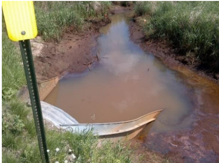
Figure 26: June 10, 2021, photo on upstream side of culvert. Showing iron in water and iron precipitate along stream edges.
