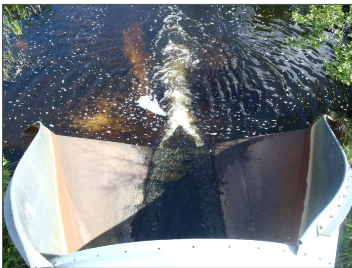
Photo 2. The downstream end of the CSAH-47 culvert. The lip of the culvert is elevated several inches above the water level in the downstream channel.
