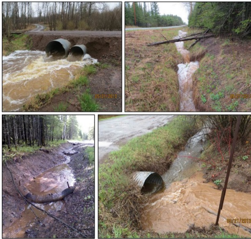
Figure 108. Examples of potential sediment sources from the road and ditch network in the Talmadge River watershed. Top left: sand and gravel entering the stream from a poorly designed road crossing. Top right: a headcut on a ditch in a neighboring watershed. Bottom left and right: water quality impacts from ditch “cleaning” efforts.
