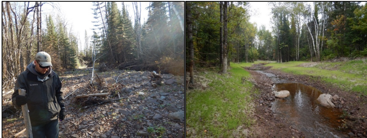
Figure 125. Before and after pictures of a stream channel/floodplain restoration project completed on the lower Talmadge River. The photo on right was taken shortly after the completion of the project. Native grasses, plants, and trees were planted in the floodplain.
