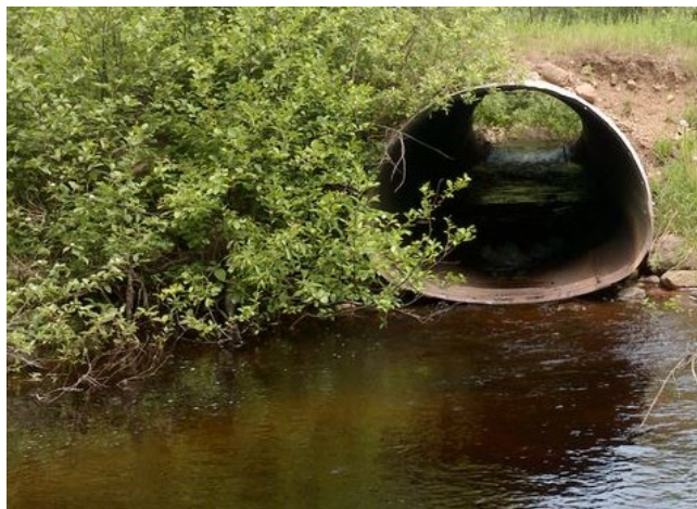
Figure 9. A perched culvert disrupting flow and fish passage on a North Shore Lake Superior tributary. Photo: Fredenberg Creek near Schroeder, MN
