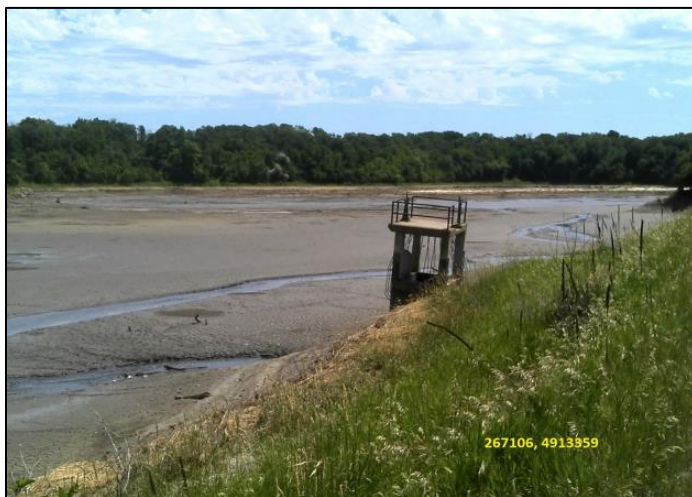
Figure 12. Brawner Lake following outlet failure (6/21/2017)
