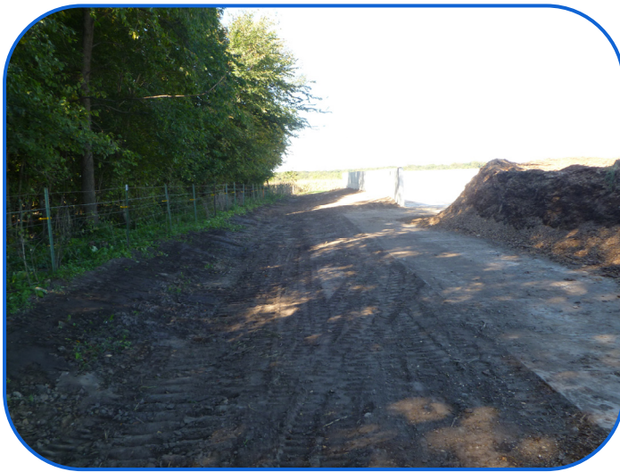
Diversion Routes Clean Water Around Feedlot
