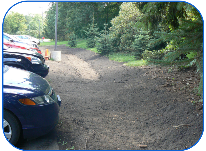
- Infiltration Trench Along a Parking Lot
