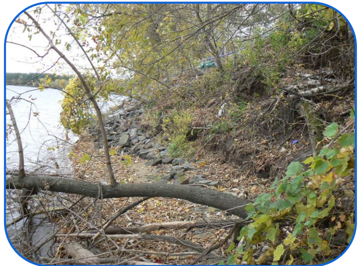
Before Shoreline Restoration – Erosion Issues
