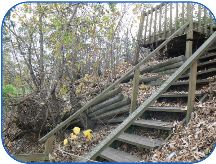
Failing Retaining Wall System
