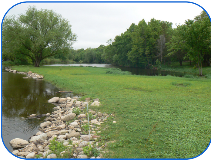
Failing Retaining Wall System
