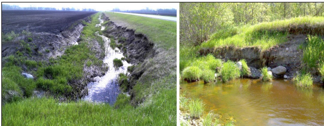
Images of sediment sources, including bank slumping along an unnamed ditch at the 200th Avenue NW and CSAH 14 intersection on May 28, 2014 (left); and streambank erosion on May 29, 2014 (right).
