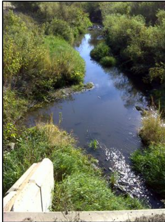
Figure 28. Sediment deposition within the culvert barrels indicate improper sizing.
