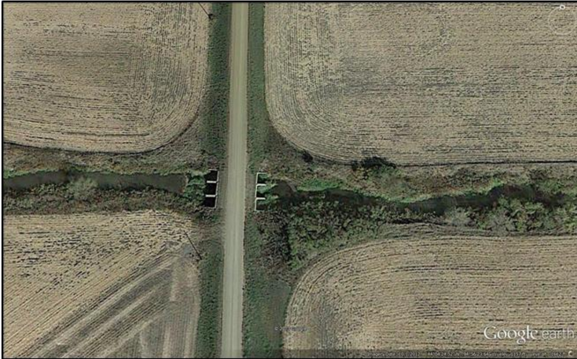
Figure 29. Triple barrel culvert, two barrels filling with sediment and providing flood plain relief during high flows.
