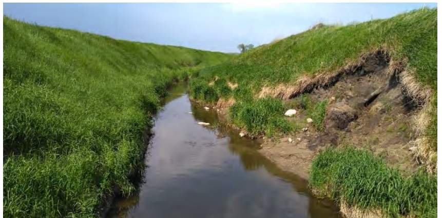
Figure 87. Photo near bio site 91MN040 showing ditch and bank erosion just downstream of a culvert.
