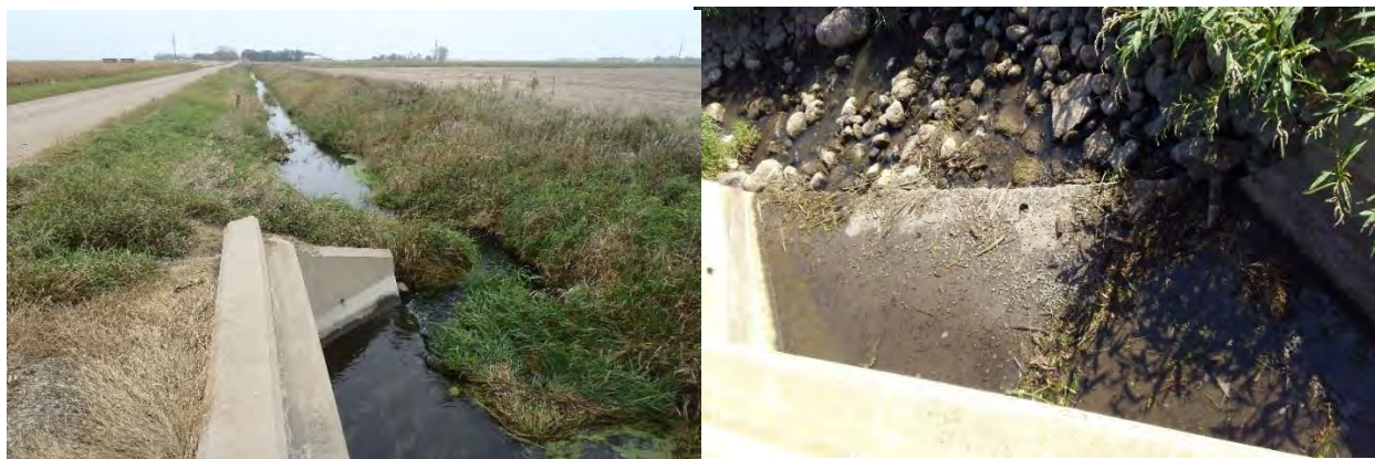
Figure 68. Photo showing both the ditched stream channel and culvert near bio site 17MN221 during fish sampling in 2017 (left). Photo of the same culvert in 2019 showing the stream water levels very low and actually flowing underneath the concrete bottom
