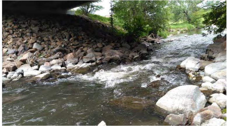
Figure 104. Photo of the artificial rapids and rip rap placed to help protect the bridge crossing near bio site 92MN047.
