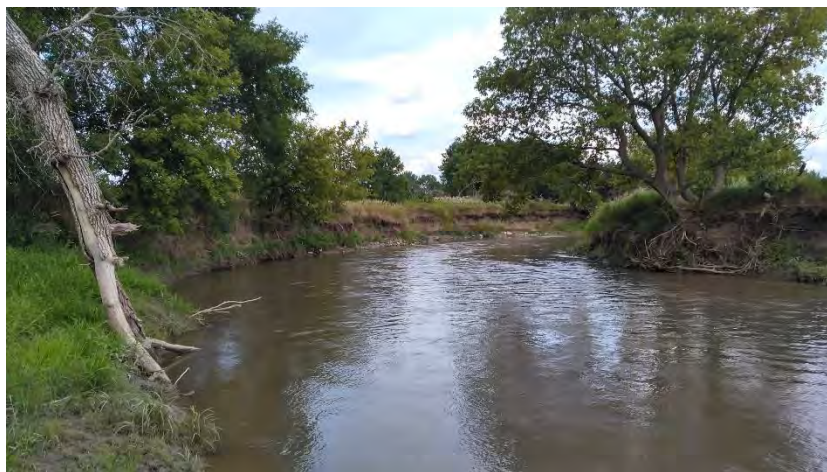
Figure 64. Photo near bio site 92MN032 showing an eroding bank.
