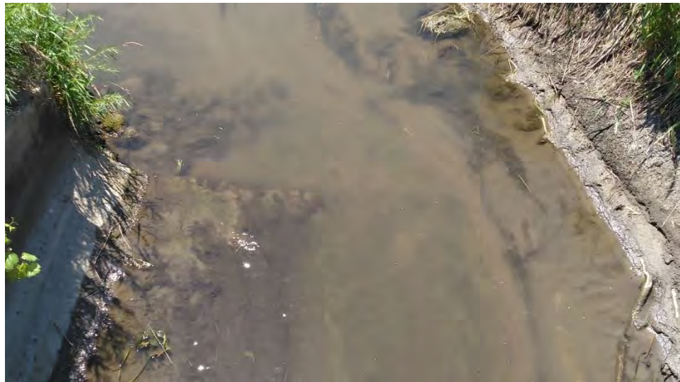
Figure 58. Photo showing the culvert near bio site 17MN215. Some dead algae lines the bottom of the culvert.
