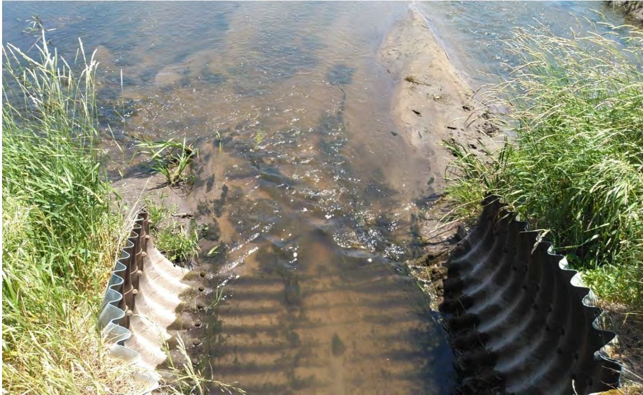
Figure 11. Photo of the culvert at bio site 17MN234 showing algae growth
