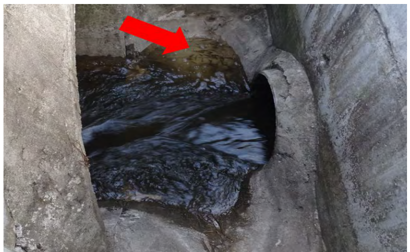
Figure 50. Road retention structure found in the upper Three Mile Creek is very likely a fish barrier.
