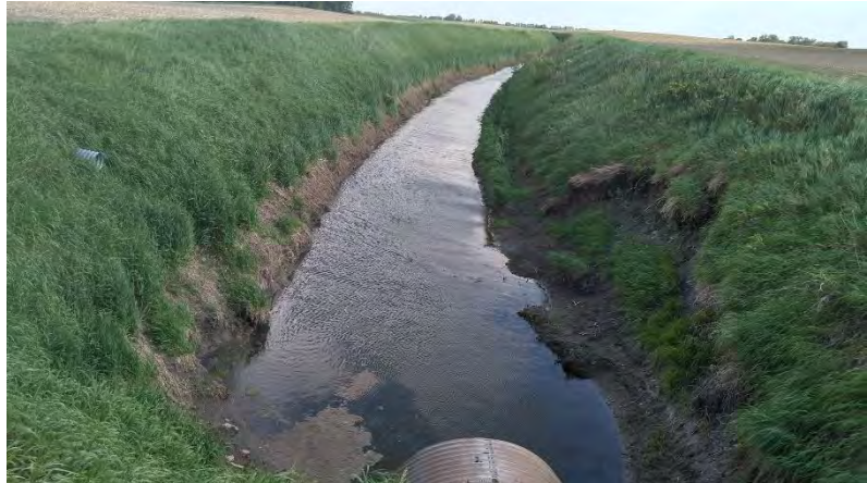
Figure 80. Photo showing the undersized culvert near bio site 17MN223.
