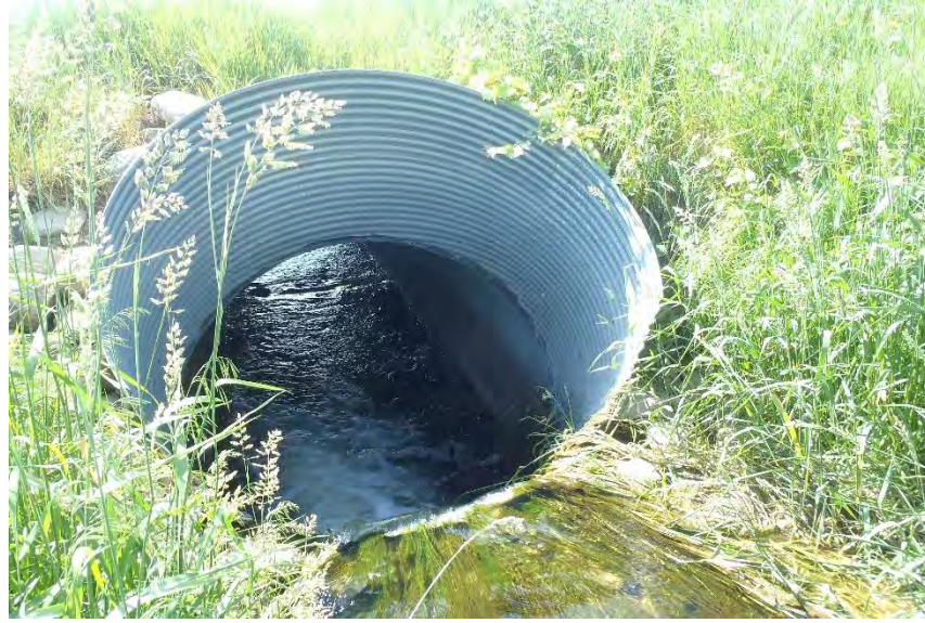
Figure 69. Photo of the perched culvert downstream of bio site 17MN221.
