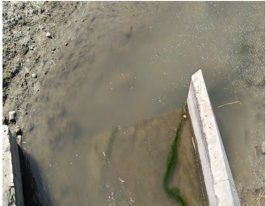
Figure 14. Photo of the culvert at the road crossing at bio site 17MN210. The bottom of the culvert appears to be at the wrong elevation compared to the bottom of the stream and could be a barrier.
