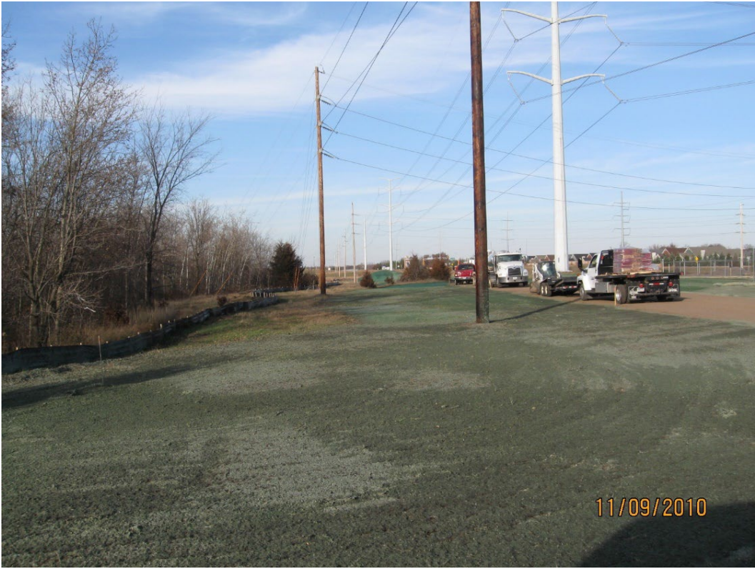
This image shows ground that has been disturbed and then stabilized with temporary hydraulically applied erosion control. This is not permanent vegetative cover and would not be acceptable.
