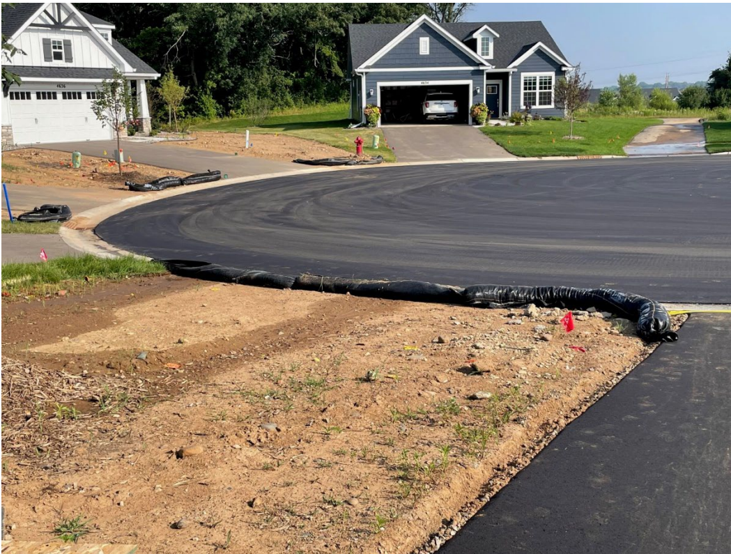
It isn't clear which lot in this residential development is being terminated. The lot in the foreground is not ready for termination.
