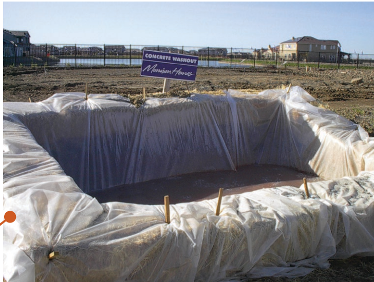
Photo 1: Well-maintained and labeled concrete truck washout
