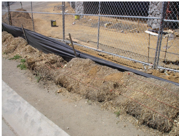
Photo 2: Hay bales and silt fence that are in need of
