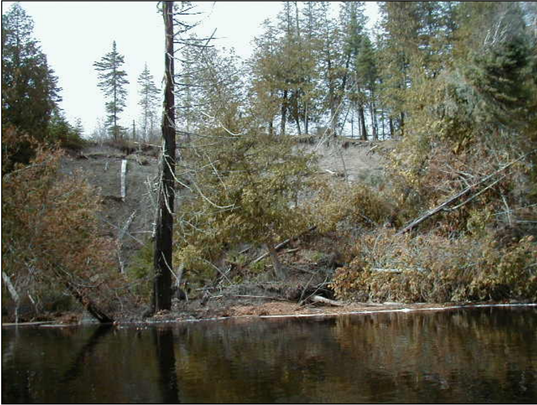
Figure 24. Streambank failure, Little Fork River, near Silverdale (Al Anderson, Minnesota DNR)
