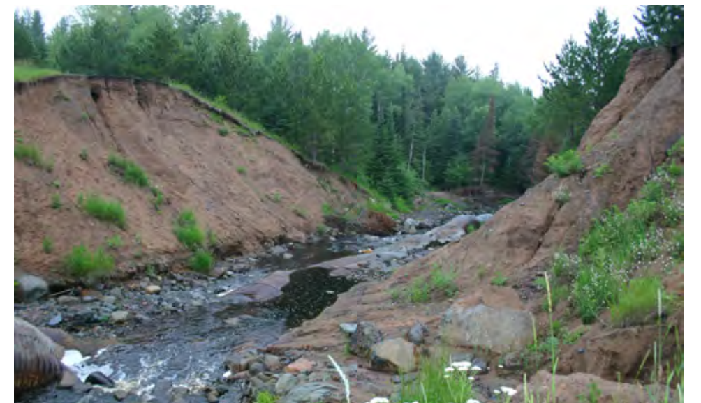
► The 2012 event also overtopped a 200 foot culvert. © Fond du Lac Resource Management Division
