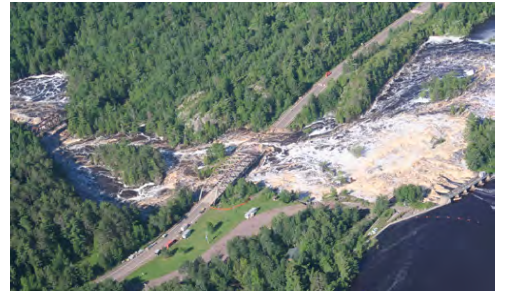
► During the 2012 event, floodwaters took out Highway 210 through Jay Cooke State Park. © Fond du Lac Resource Management Division
