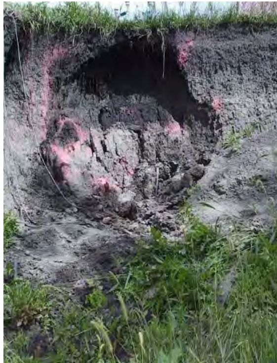
Figure 11. Picture of the bank along the Le Sueur River after a rotational failure due to pore water pressure build up behind it.
