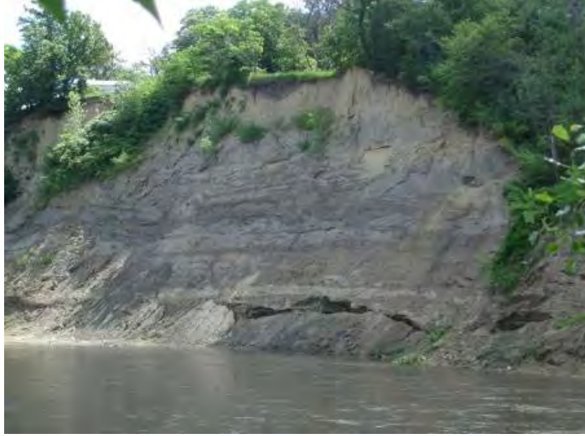
Figure 13. A picture of the slumping bank along the Blue Earth River, MN. The slump is caused by detachment of the bank bottom due to low soil strength and heavy wet soil during recession hydrograph.
