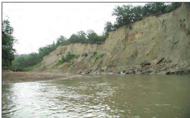
Fig. 2. A steep tall bank actively sloughing along the Le Sueur River in Blue Earth County, Minnesota. Accumulated material at the toe is from past bank sloughing from above. Lack of vegetation on part of the bank indicates active sloughing nature of this bank.
