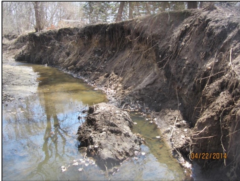
Figure 11. Streambank erosion in Coon Creek Subwatershed.
