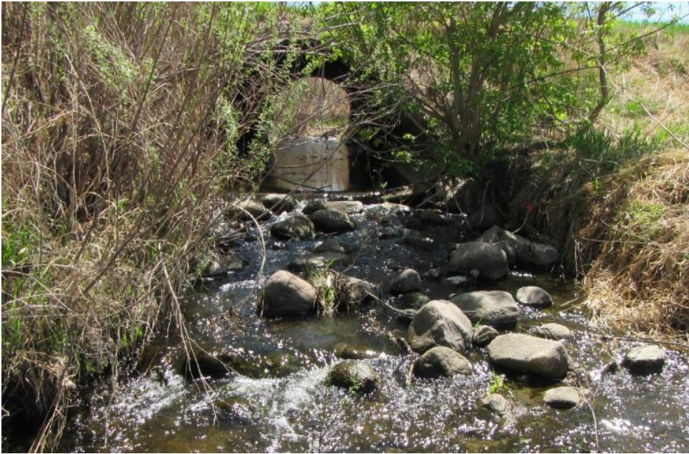
Figure 50. Perched culvert downstream of 380th Street.
