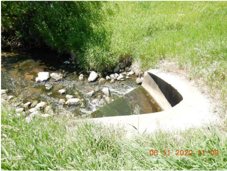
Figure 5. Perched Culvert off CR 73 NE, on AUID -637.
