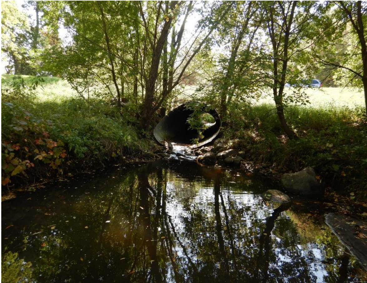
Figure 104. Sour pool, downstream of 260th Street.
