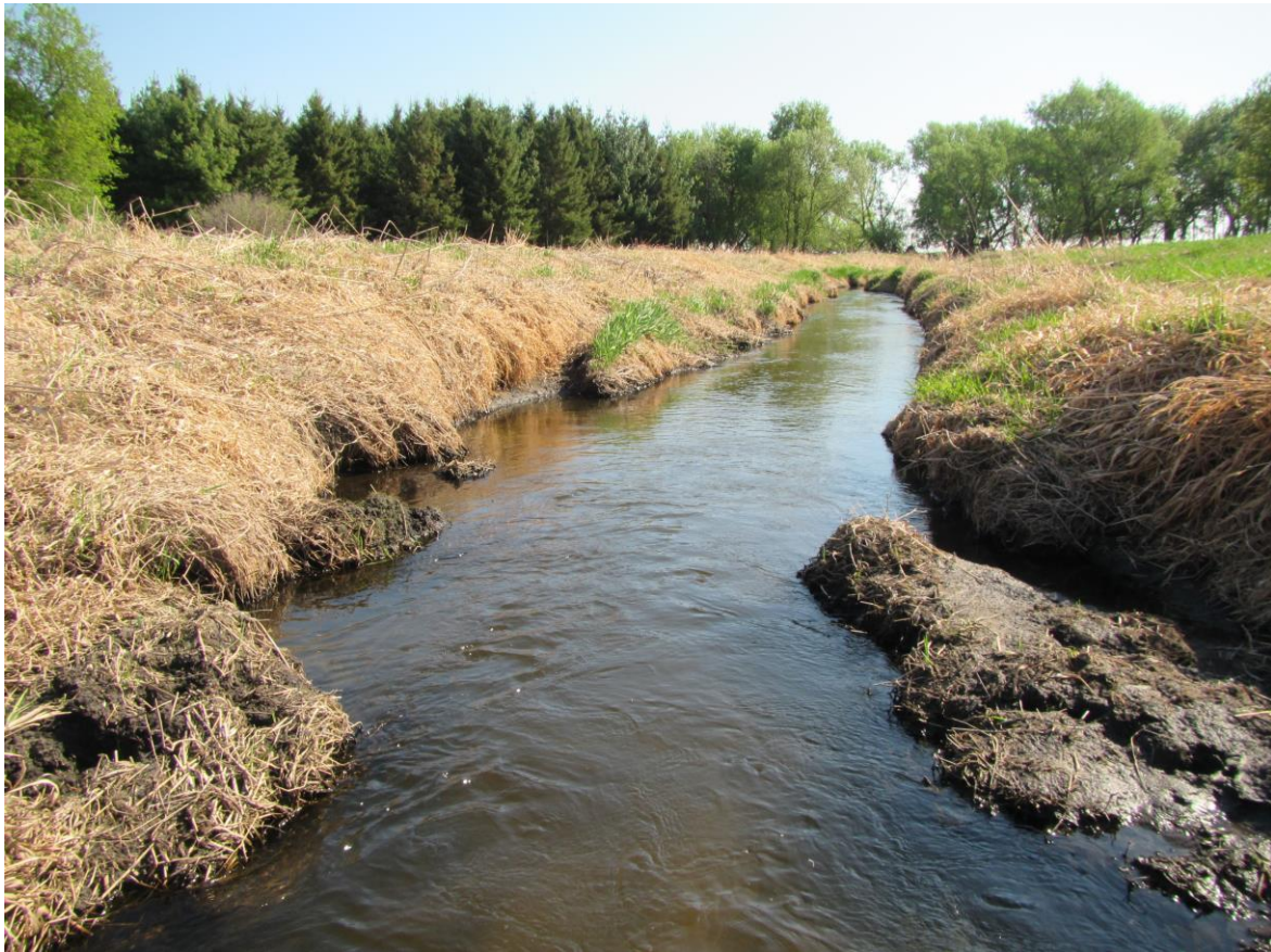
Figure 36. Bank failure in the upstream portion of Unnamed Creek, spring 2018.
