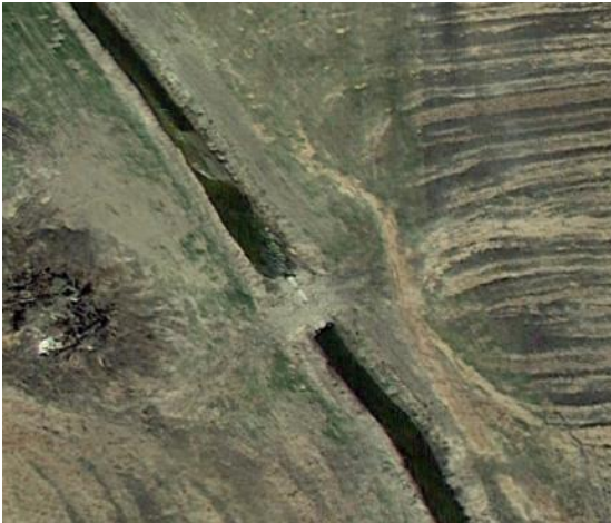
Figure 51. Field crossing with poorly placed culvert on Unnamed Creek.
