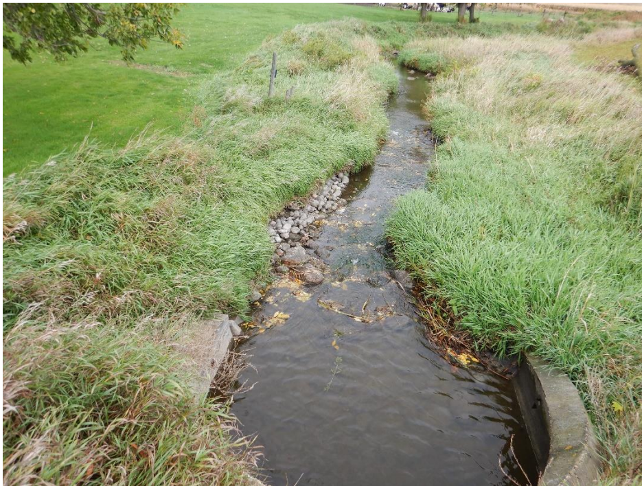
Figure 30. Boulders and cobbles acting as a grade control, downstream of CR 91.
