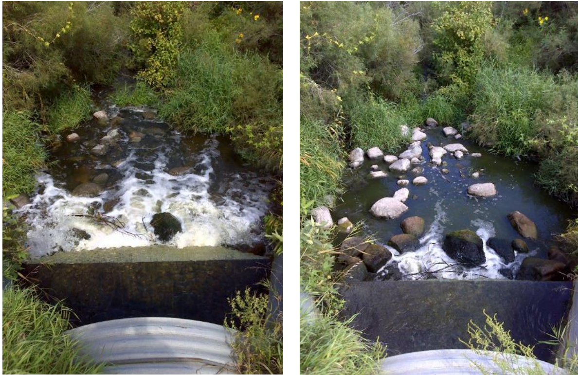
Figure 54. Perched culvert off 380th Street is a barrier at moderate (left) and low (right) flow.
