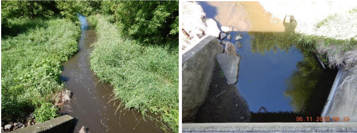
Figure 94. Suspended sediment after a storm event, and the resulting plugging of the culvert.
