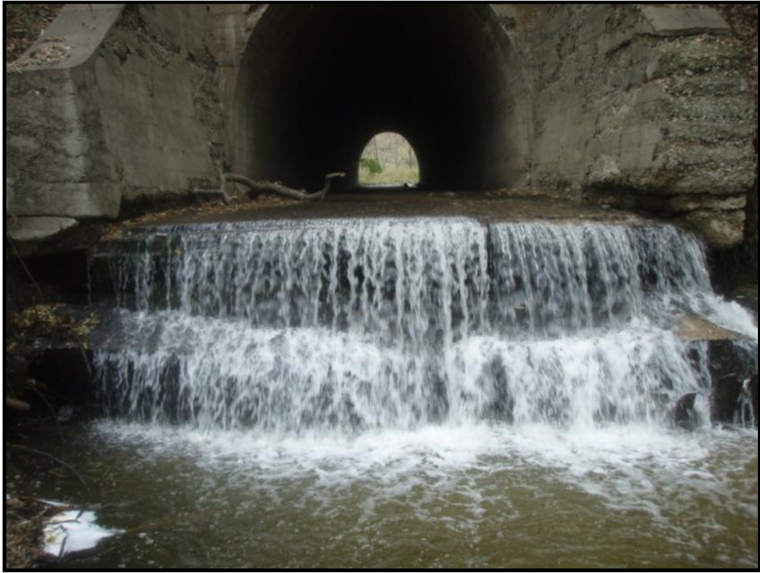
Figure 4.7 Large drop at downstream end of regional trail culvert (looking upstream)
