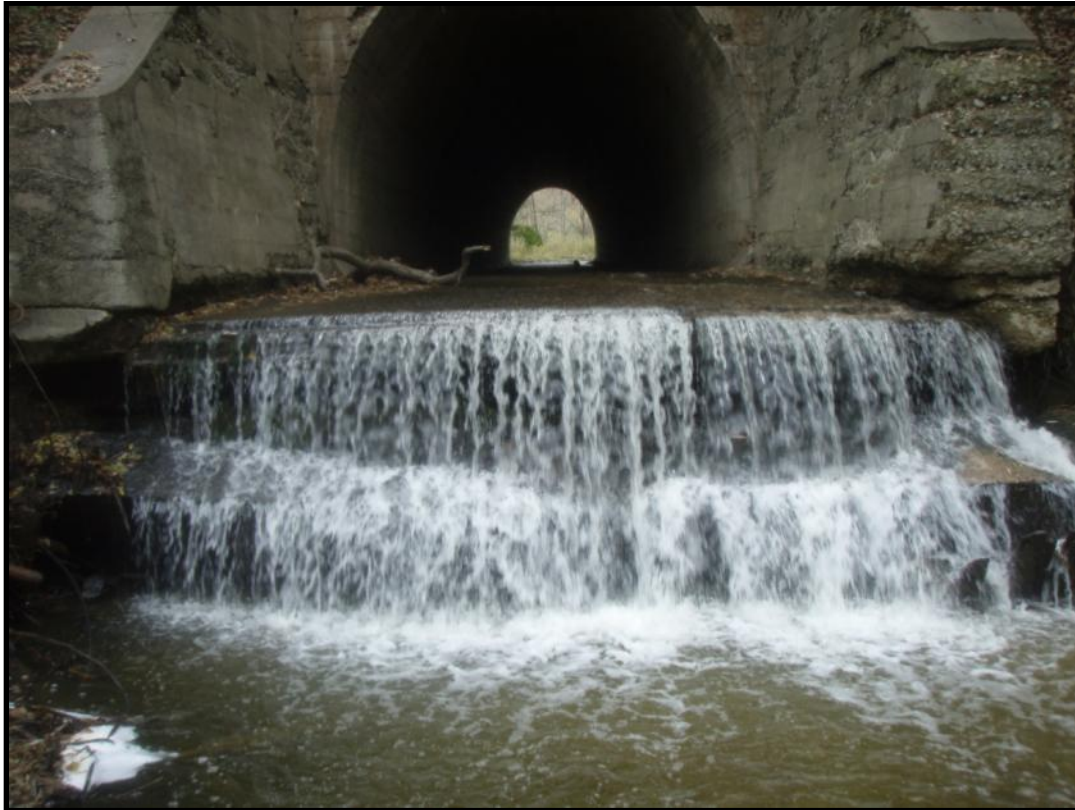
Figure D.7 Large drop at downstream end of regional trail culvert (looking upstream)
