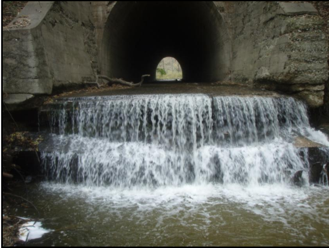
Figure 3.1 Large drop at downstream end of regional trail culvert (looking upstream)
