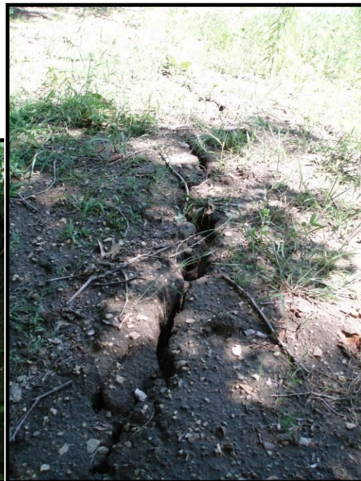
Figure 4.15 Crack foretelling impending slope failure (Site 7)
