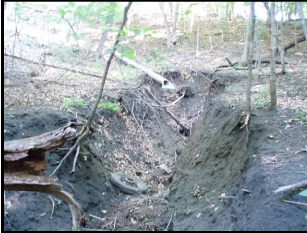
Figure 4.4 Large Headcut in Main Ravine Below Pipe Outlet from Mandan Circle (Site 2)
