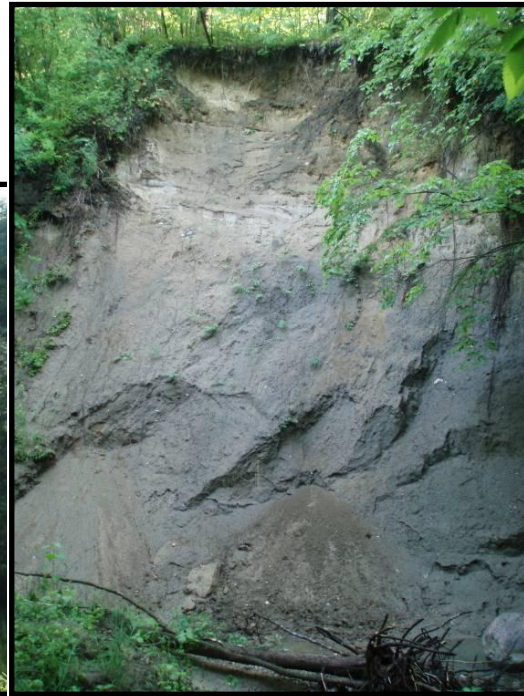
Figure 4.23 Bank failure on creek (Site 11)
