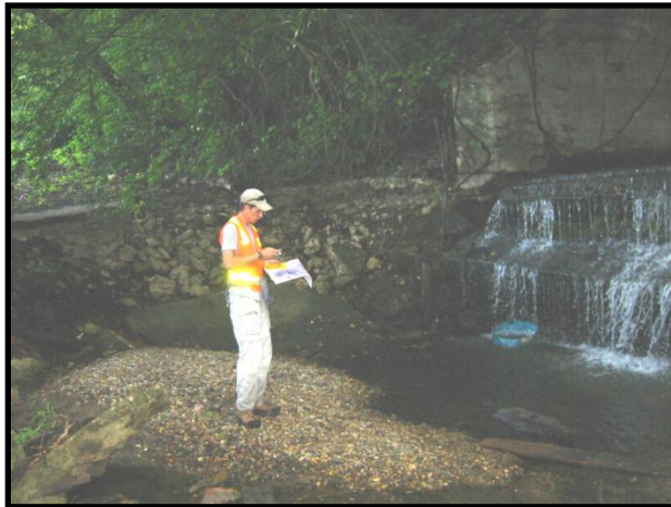
Figure 4.2 Large drop and undermining at downstream end of regional trail culvert (Site 1)
