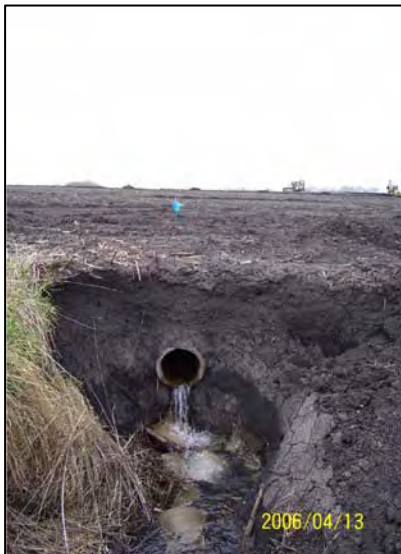
Systems that discharge partially or untreated sewage directly to surface water are often referred to as “straight pipe septic systems”.
