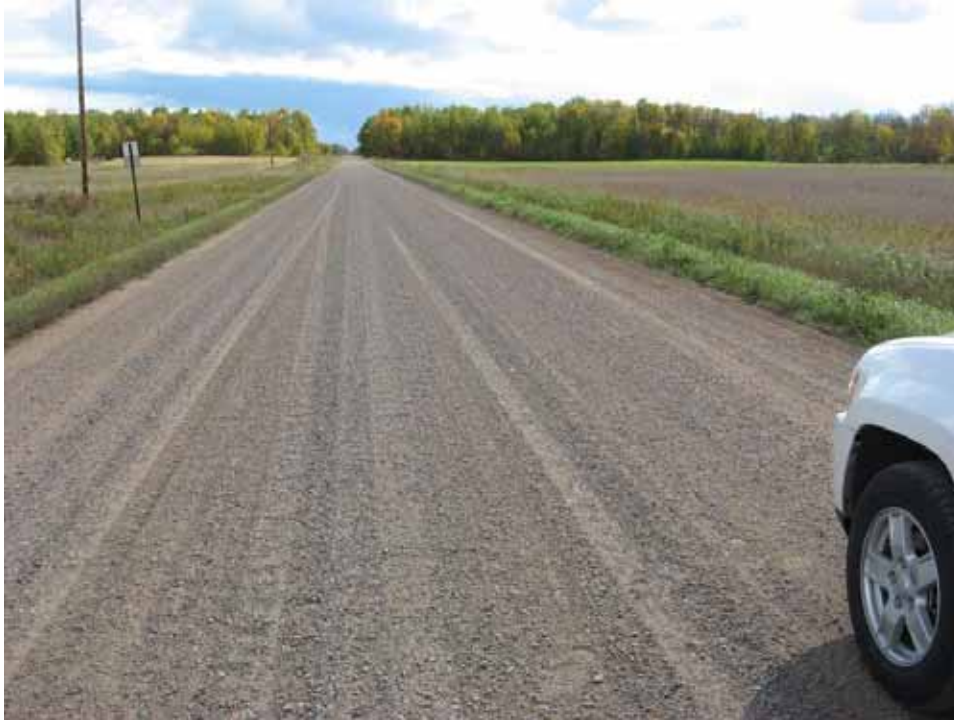
Another example of graveled road cover, approximately 25-feet wide, crowned, and bladed in the previous few days – possibly move picture.
