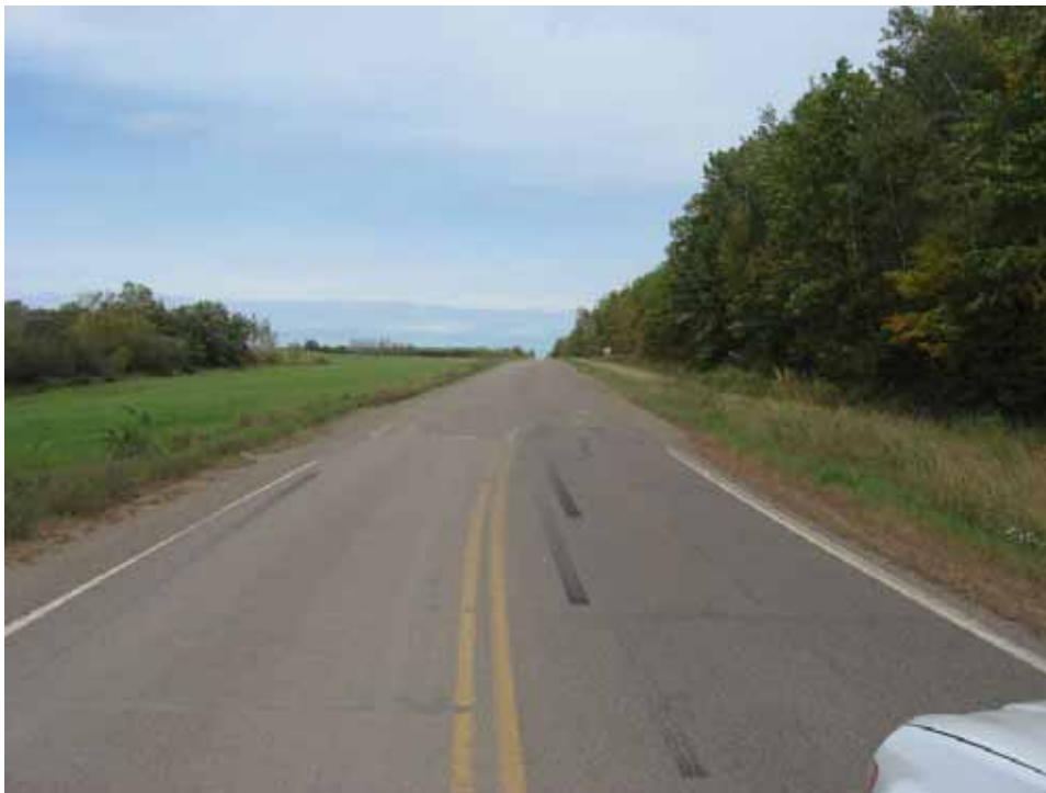
Transition from asphalt paved road to graveled road near the intersection of Hwy 10 and 170 th Avenue. In general the gravel roads were very well maintained and no evidence of sediment input at stream crossings was observed. Roadside ditches were not common.
