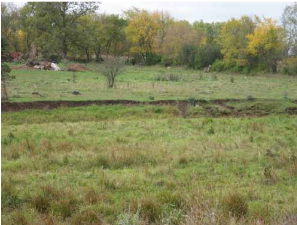
Close-up of streambank slumping. Based on the knickpoint at the top of the streambank and the grass on the streambank, it is clear the toe of the streambank is being eroded and the upper bank slumps into the river.
