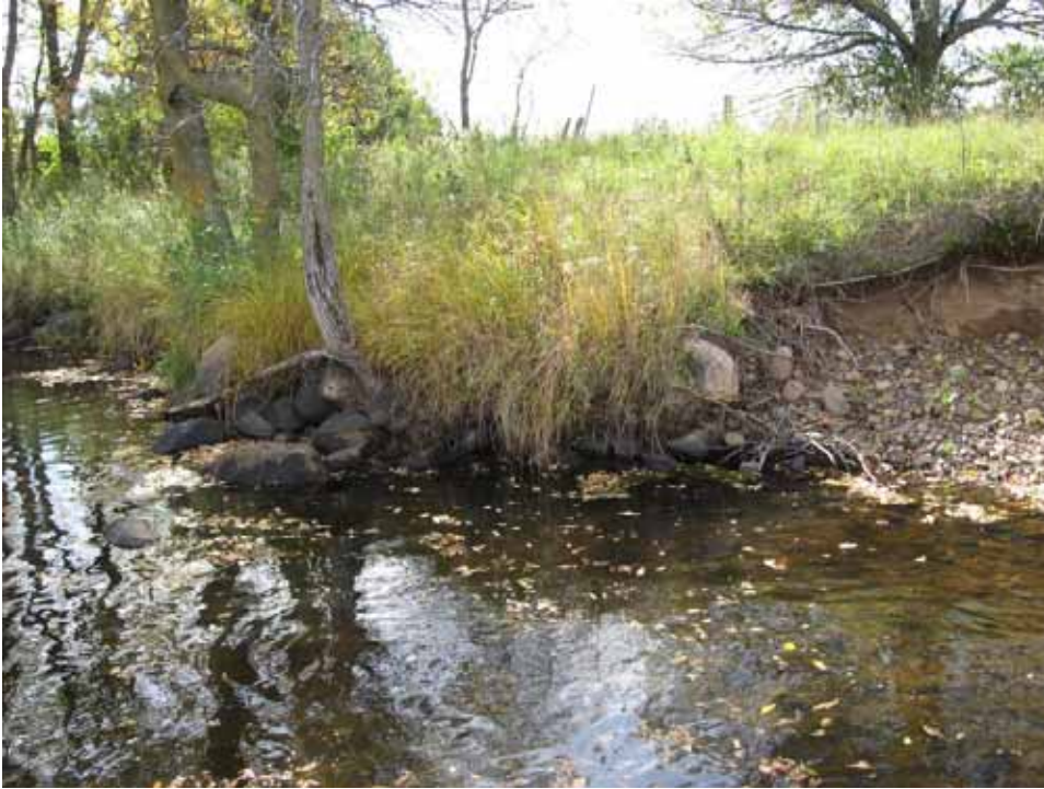
Downstream view of right bank at the head of a bend. The boulders to the left of the photo were likely placed by the adjacent landowner to minimize streambank erosion. Note the contrast with the upstream conditions where no boulders were installed.
