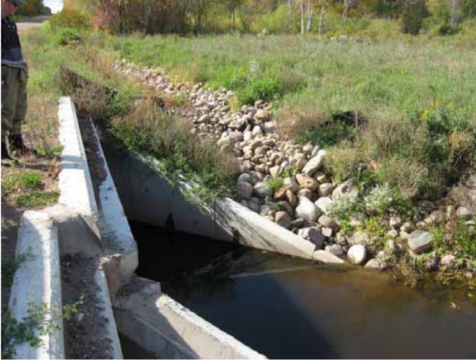
View of roadside drainage ditch entering the South Fork from CR-49. The depositional fan at the toe of the riprap ditch indicates the graveled road surface does contribute some fine material to the system.
