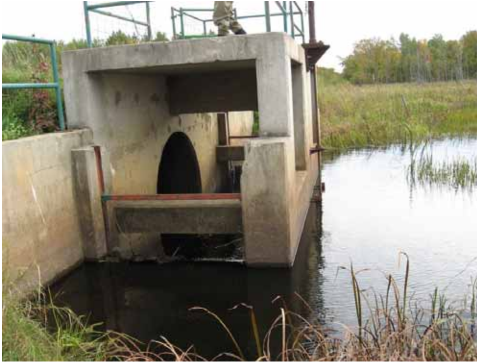
Control structure used to maintain the water surface elevation of the impounded area shown in the previous photograph. The culvert barrel is a CMP 8-feet in diameter.
