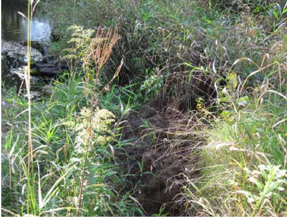
View of the block failure shown in previous photos as seen from the top of the bank.
