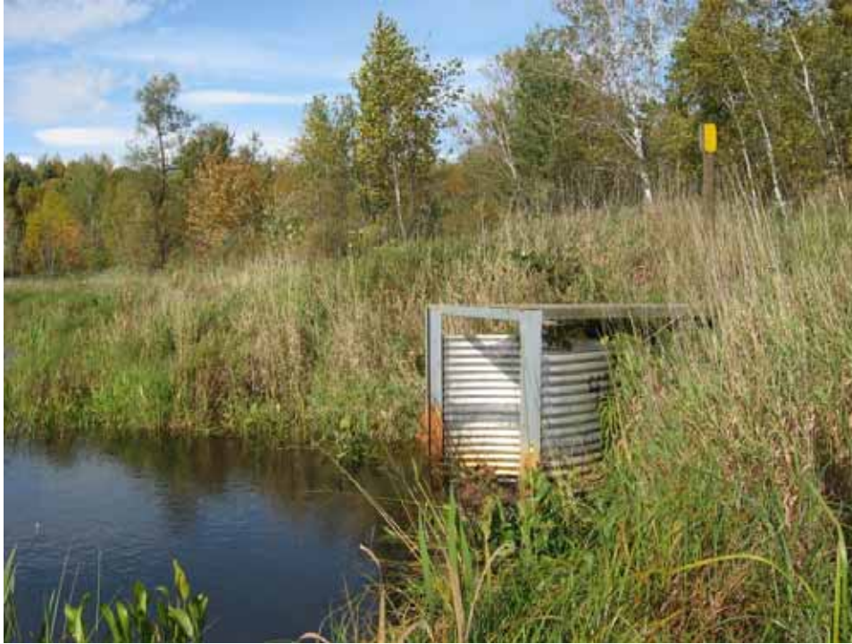
Flashboard riser structure to control flows from a large lake/wetland to a small tributary to the Groundhouse that enters just downstream of the site visited off of Apple Road.
