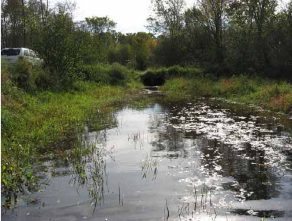
Downstream view from of the “wetland flowage” shown in the previous photo. A culvert crossing is located near the vehicle on the left bank.
