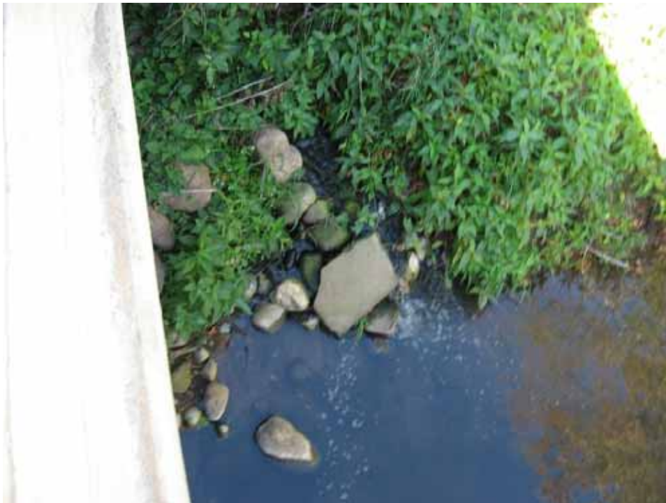
Outfall from the Ogilvie publicly owned wastewater treatment works (POTW) located on the right streambank immediately upstream of the Hwy 23 crossing. No changes in water quality were observed downstream of the outfall.
