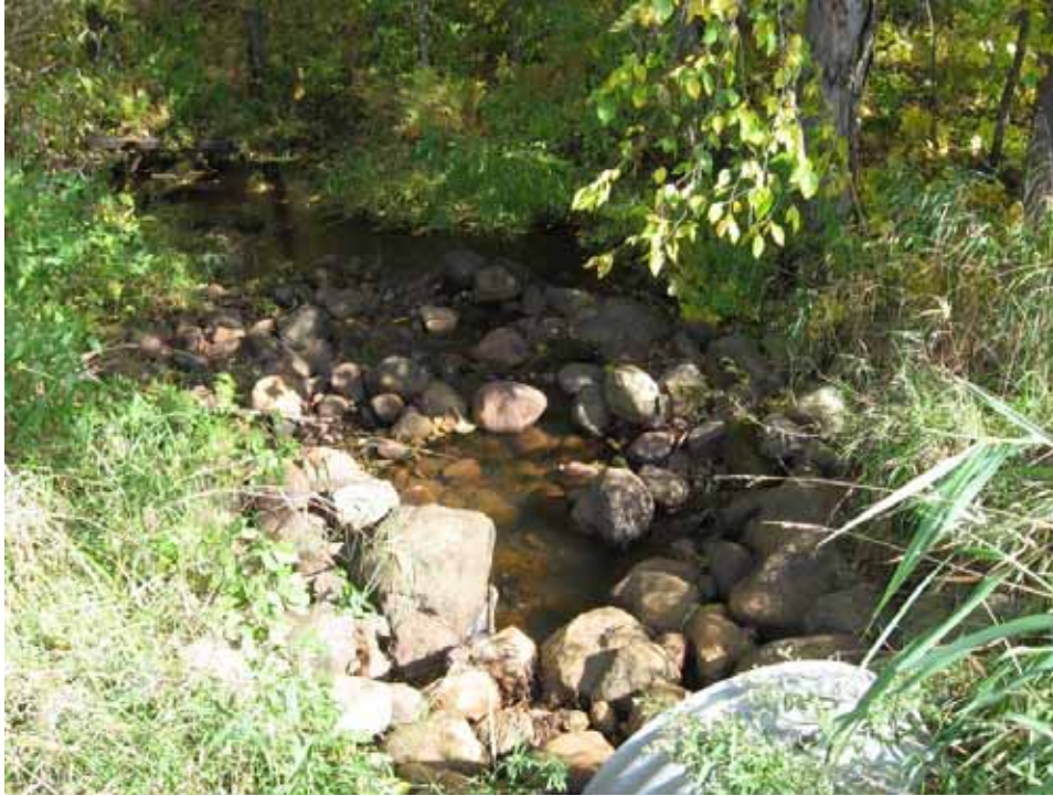
Downstream end of the culvert from the outlet structure shown in the previous photographs. The 36-inch CMP discharges to placed riprap before entering the small tributary.
