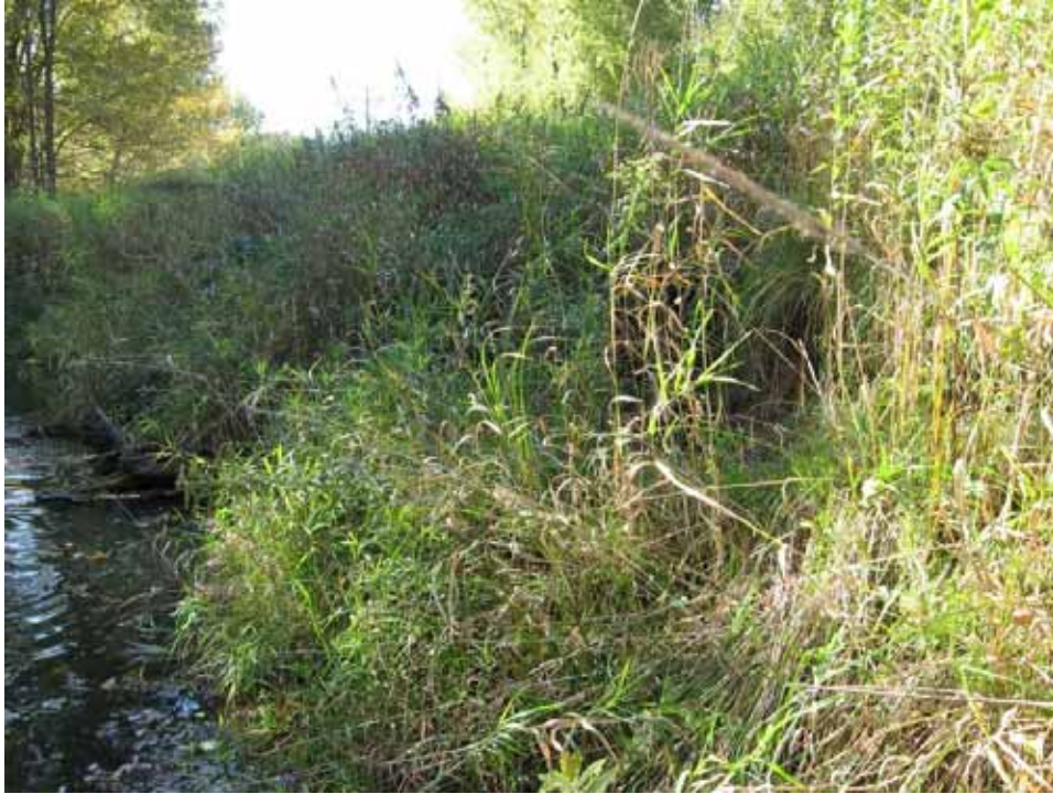
Close up view of large block of streambank material detached from the streambank. The location along the power line corridor indicates the lack of woody vegetation contributes to the susceptibility of the streambanks to destabilizing forces.
