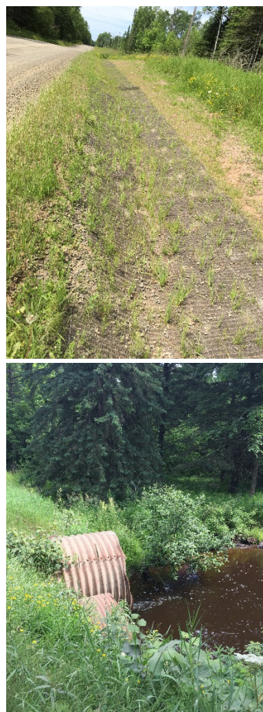
Figure 24. Top: Restored ditch lacking established vegetation; Bottom: Culvert identified as fish passage barrier.
