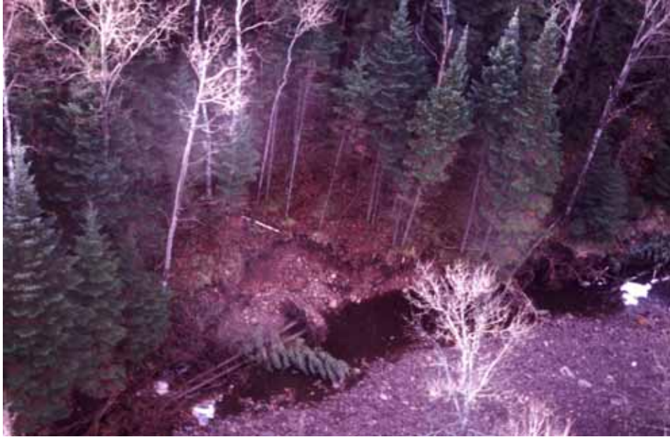
Figure 3.12. Example of mild bank erosion.
