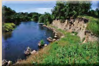
Root wad revetment and a revegetated bankfull bench built to stabilize a cutbank encroaching on Interstate 94, two years after construction (looking downstream).
