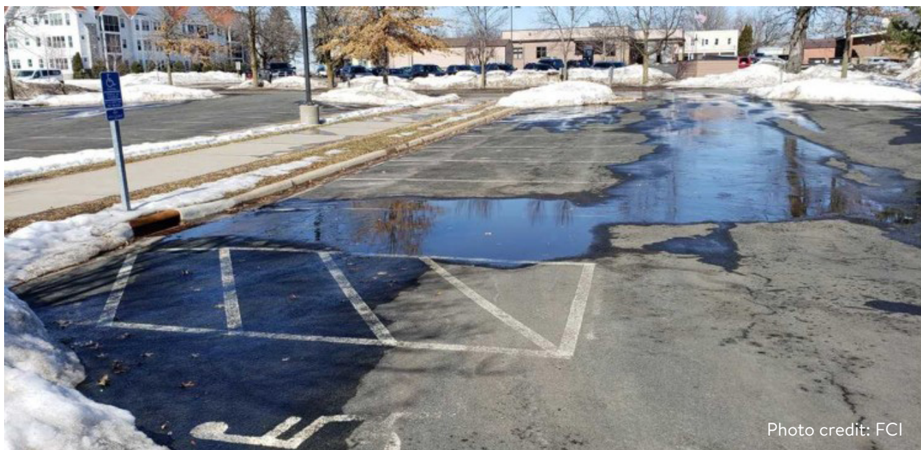
Figure 4-8 Example of improper snow storage. Melt water coming from snow piles will freeze creating a slippery parking lot.
