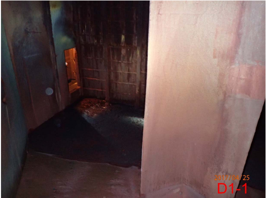
Photo 88 Base of Stack D (8)
