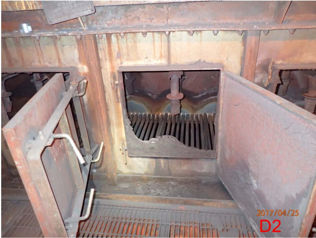
Photo 99 Scrubber D Mid-body (6)
