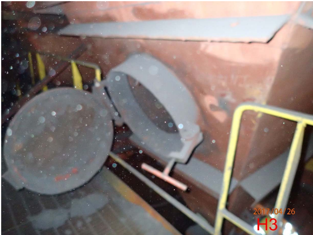
Photo134 Multiclone Cones at Second Level (7)
