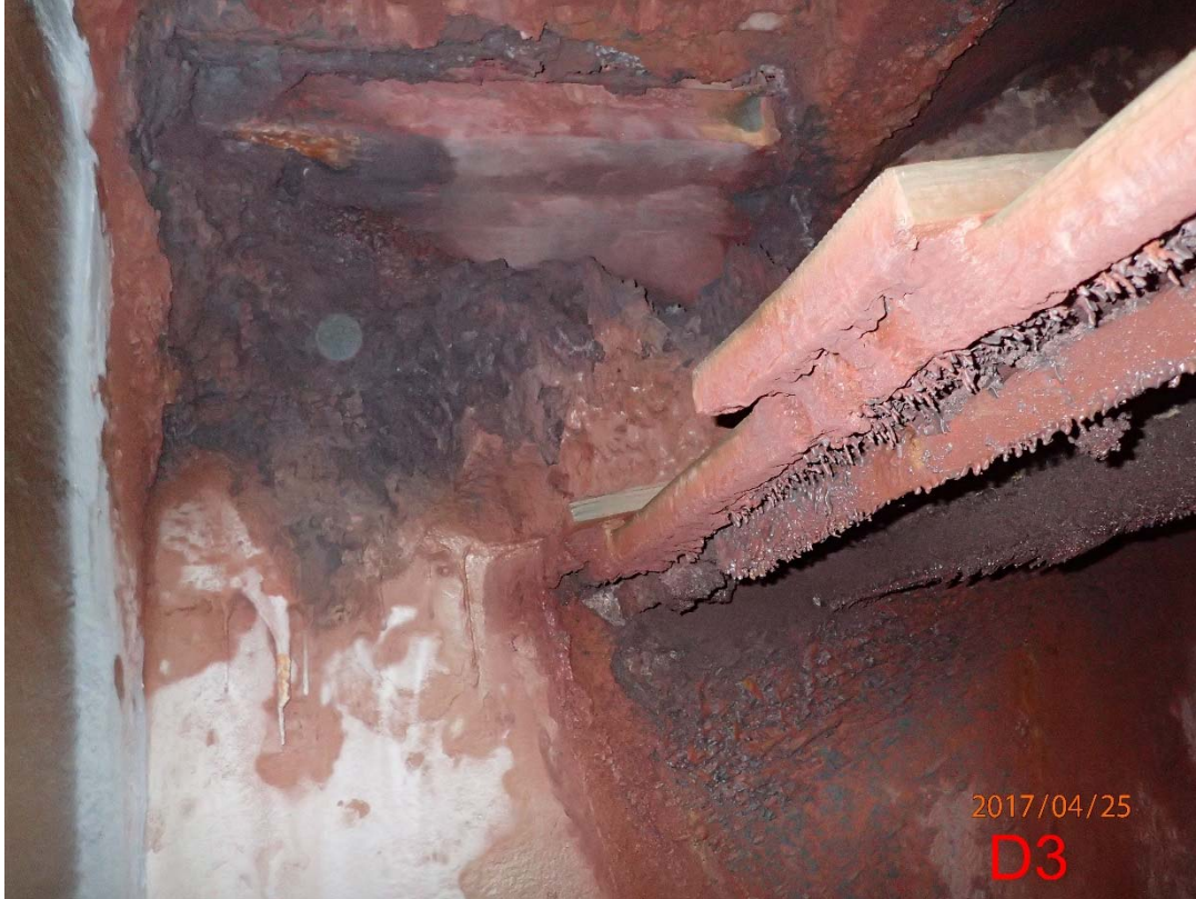
Photo 107 Scrubber D Lower-body (4)
