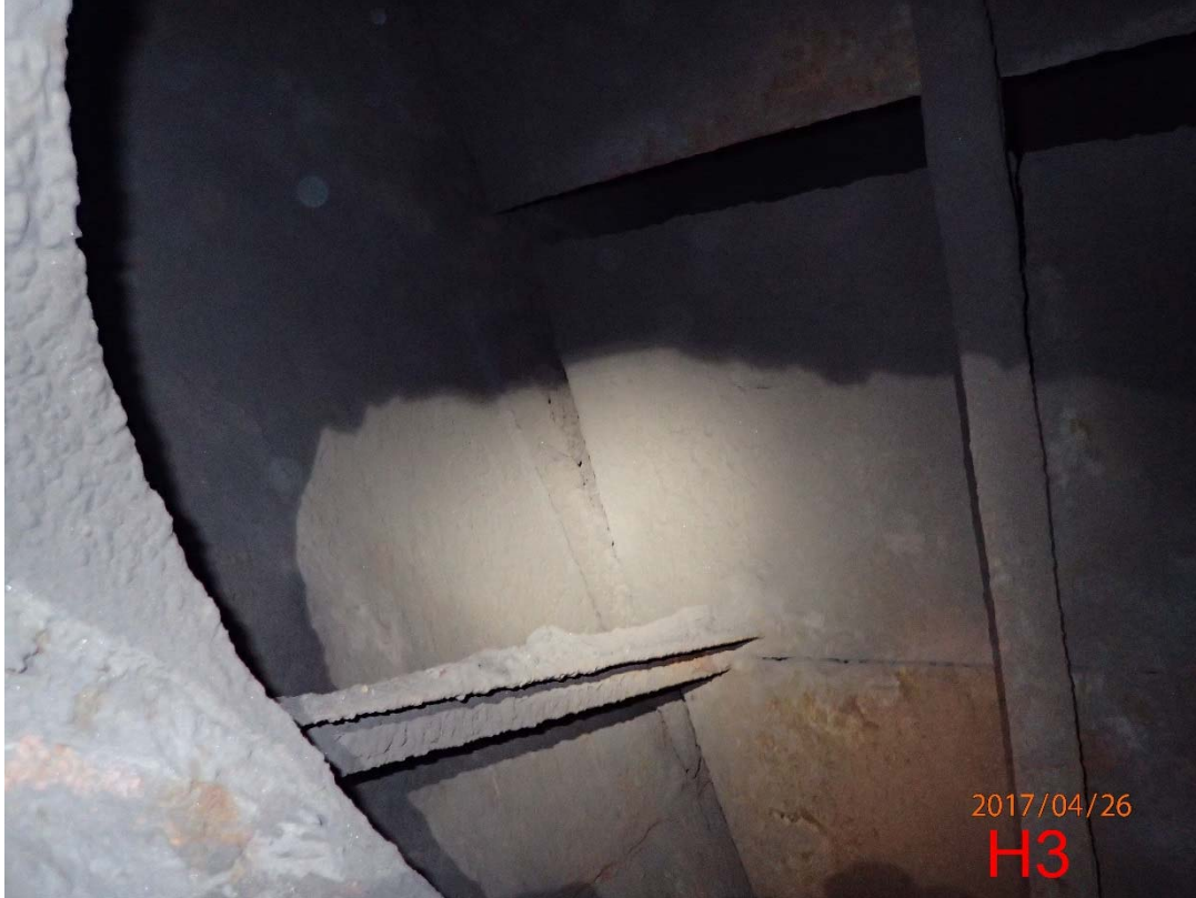
Photo 129 Multiclone Cones at Second Level (2)
