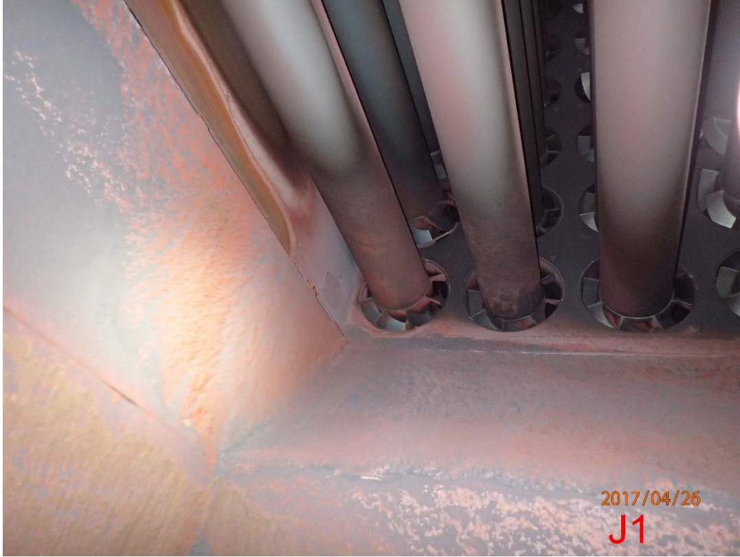
Photo 161 Ducting off Process Gas Header (8)
