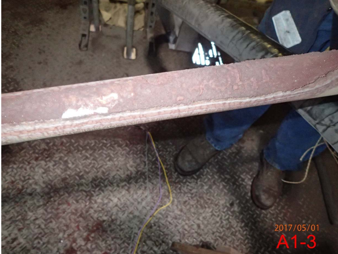
Photo 11 Stack A CEMS Probe (2)
