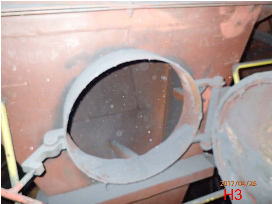
Photo 142 Multiclone Cones at Second Level (15)
