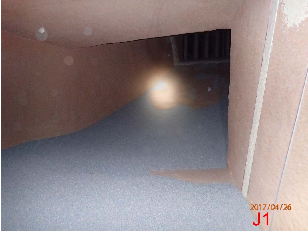
Photo 159 Ducting off Process Gas Header (6)
