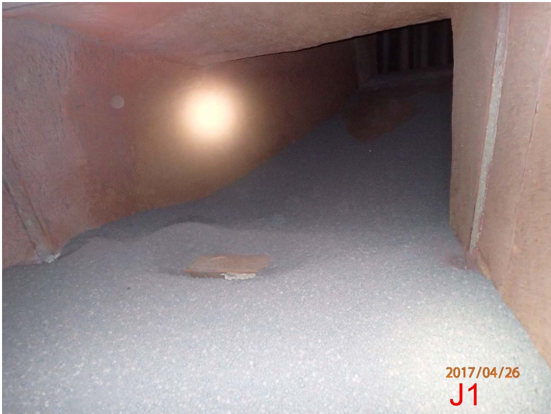
Photo 156 Ducting off Process Gas Header (3)
