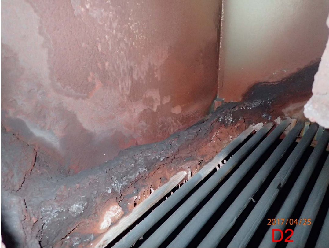
Photo 101 Scrubber D Mid-body (8)
