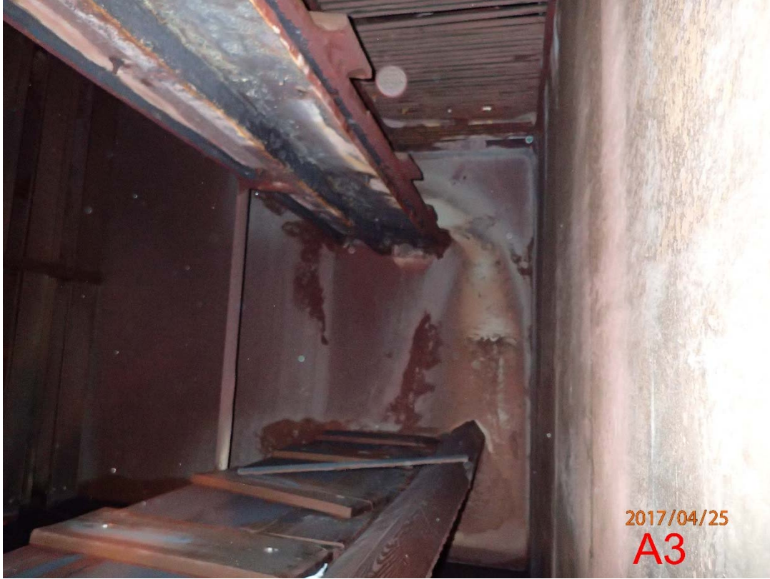
Photo 21 Scrubber A Lower-body (2)
