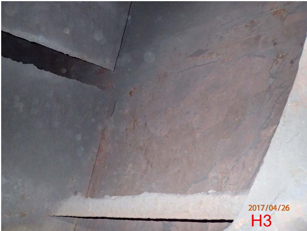
Photo 130 Multiclone Cones at Second Level (3)
