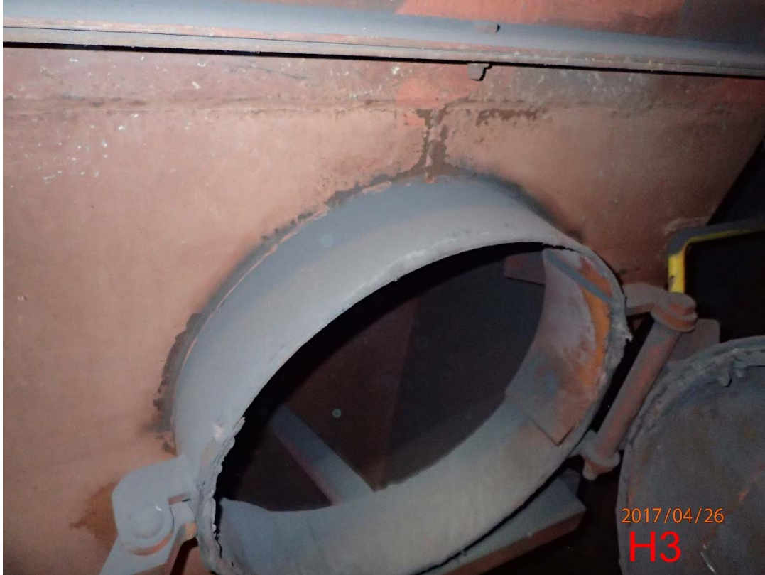
Photo 143 Multiclone Cones at Second Level (16)
