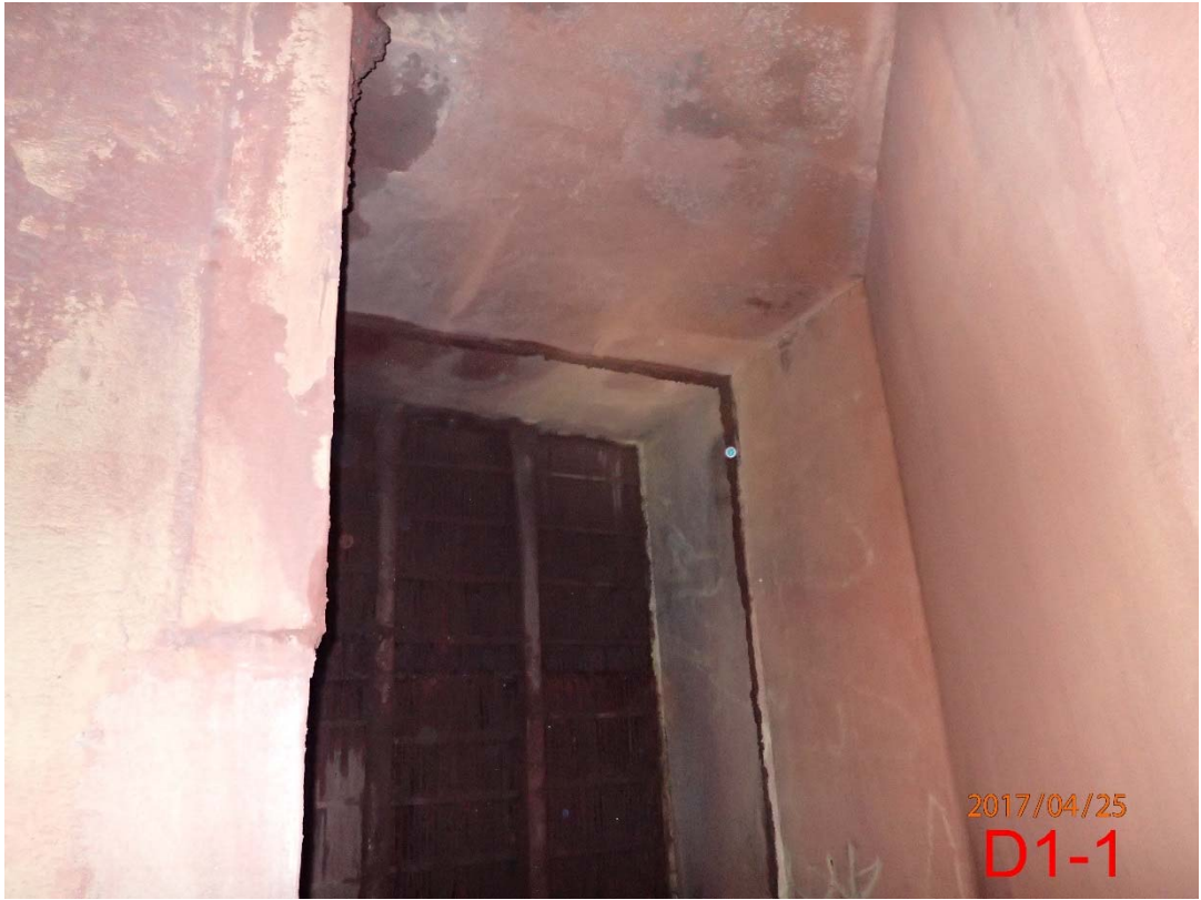
Photo 86 Base of Stack D (6)
