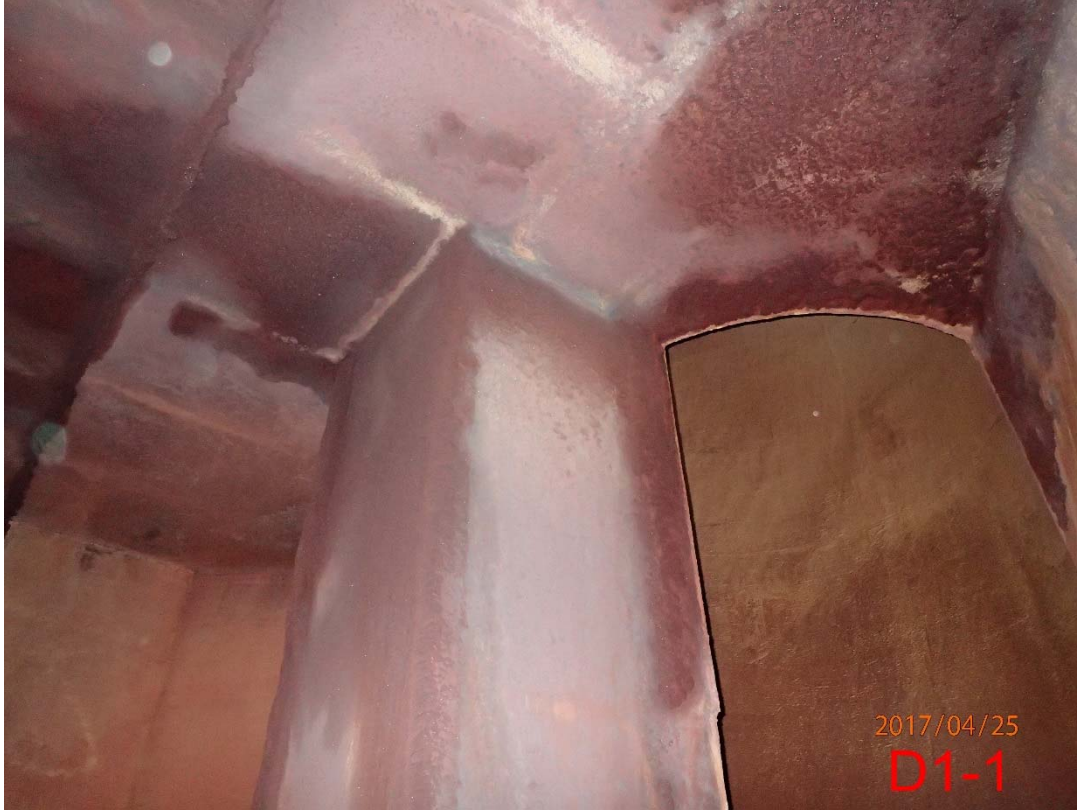
Photo 83 Base of Stack D (3)
