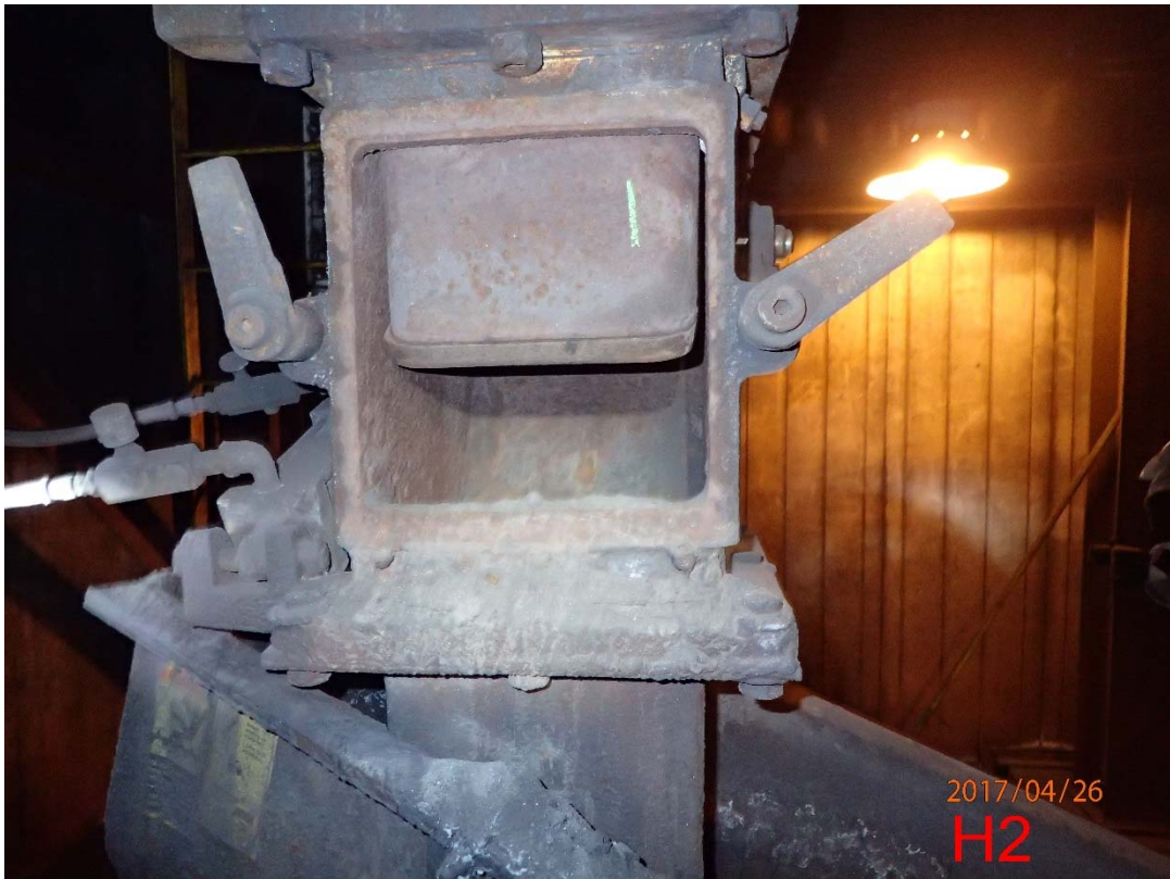
Photo 120 Multiclone Cones Discharge at Ground Level (1)
