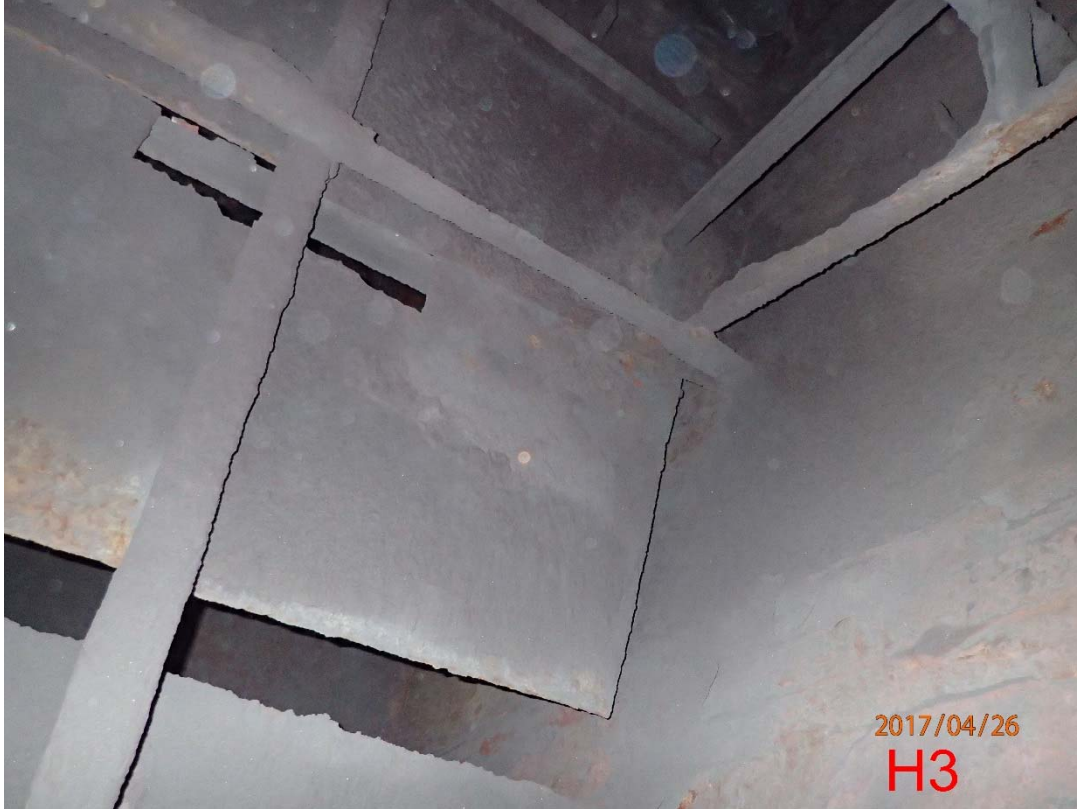
Photo 133 Multiclone Cones at Second Level (6)
