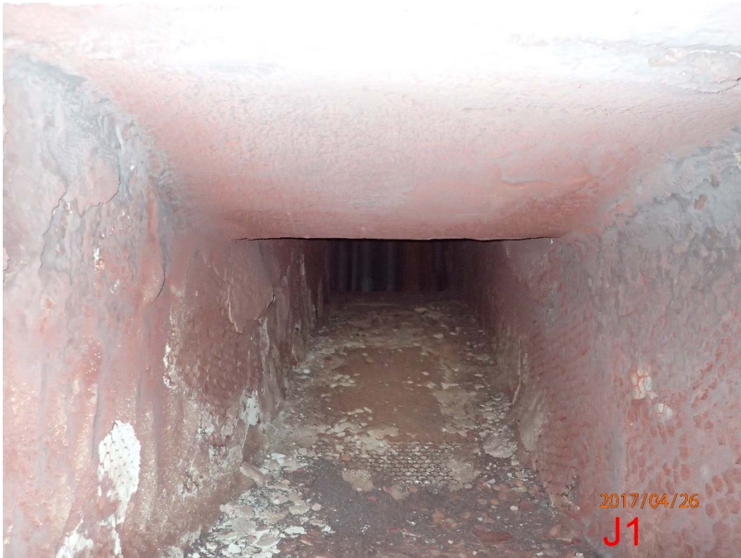
Photo 154 Ducting off Process Gas Header (1)
