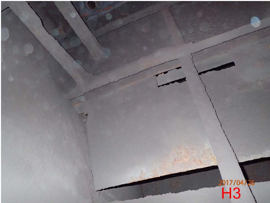
Photo 132 Multiclone Cones at Second Level (5)
