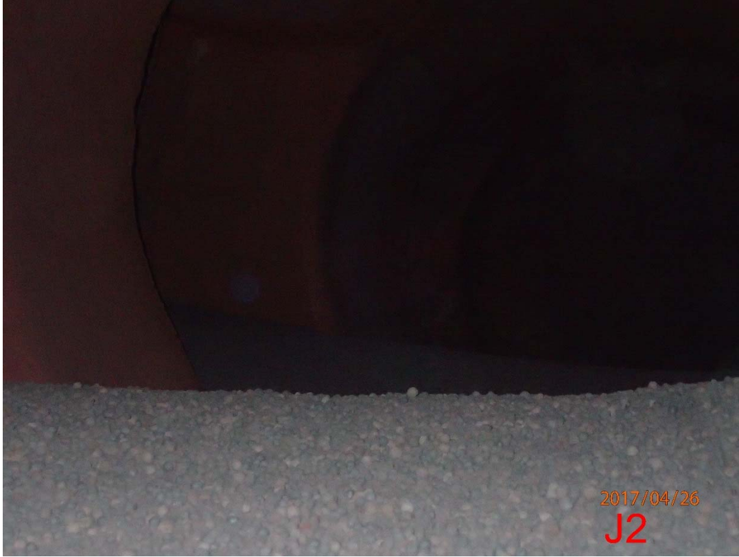
Photo 165 Access of Process Gas Header (2)
