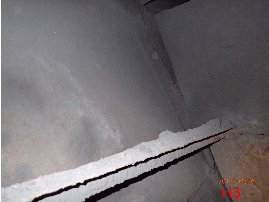
Photo 131 Multiclone Cones at Second Level (4)
