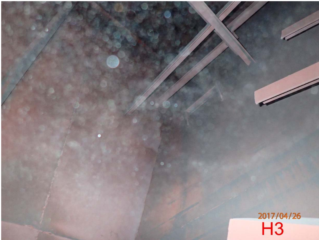
Photo 138 Multiclone Cones at Second Level (11)
