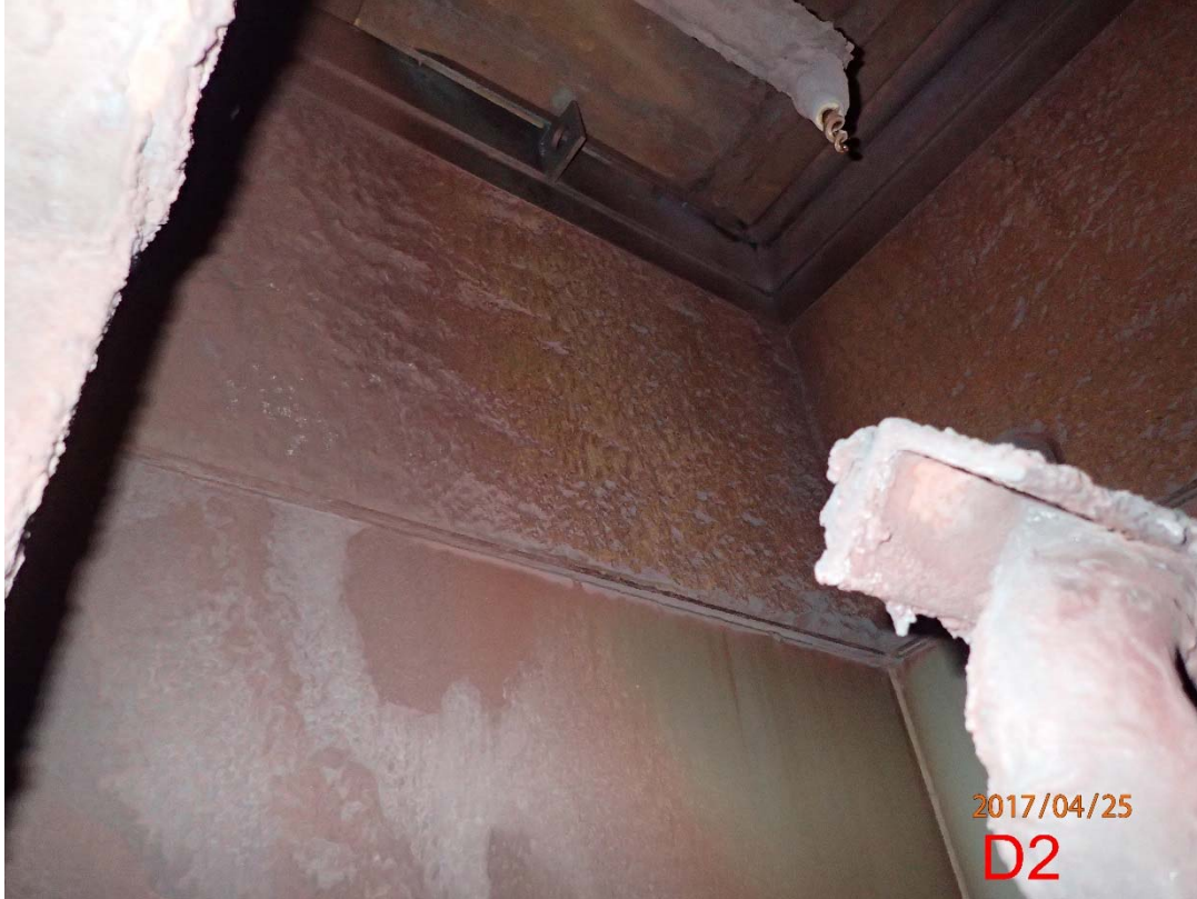
Photo 103 Scrubber D Mid-body (10)
