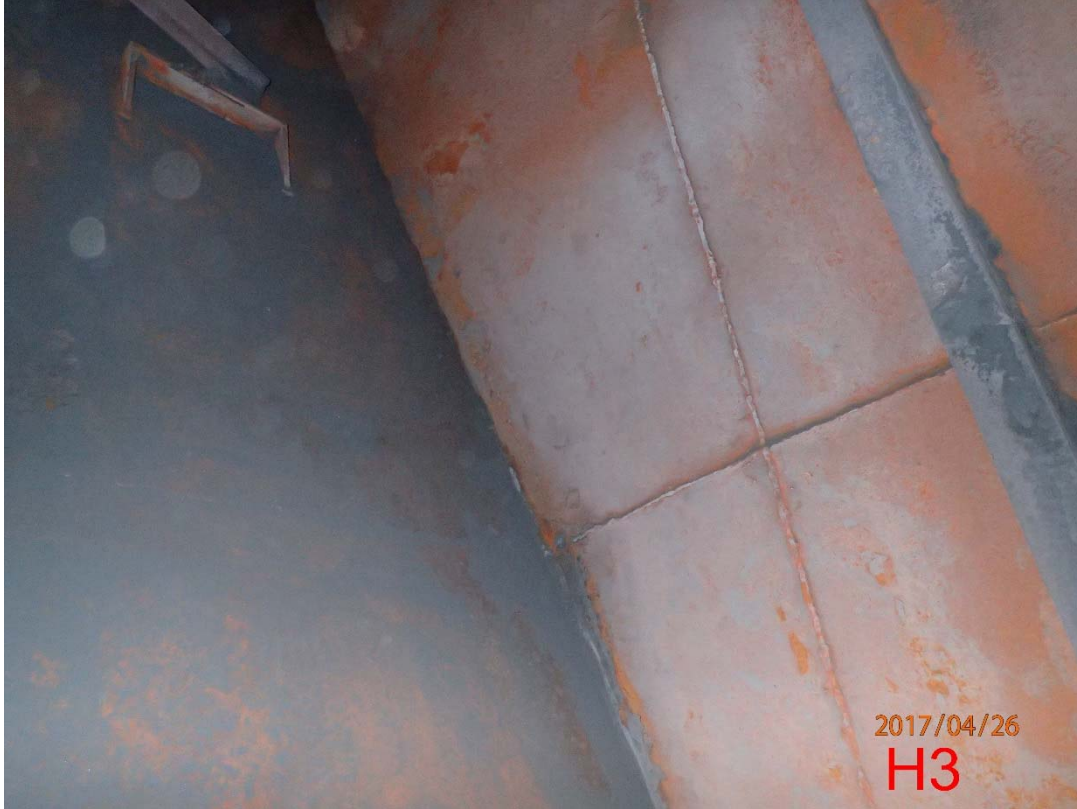
Photo 135 Multiclone Cones at Second Level (8)
