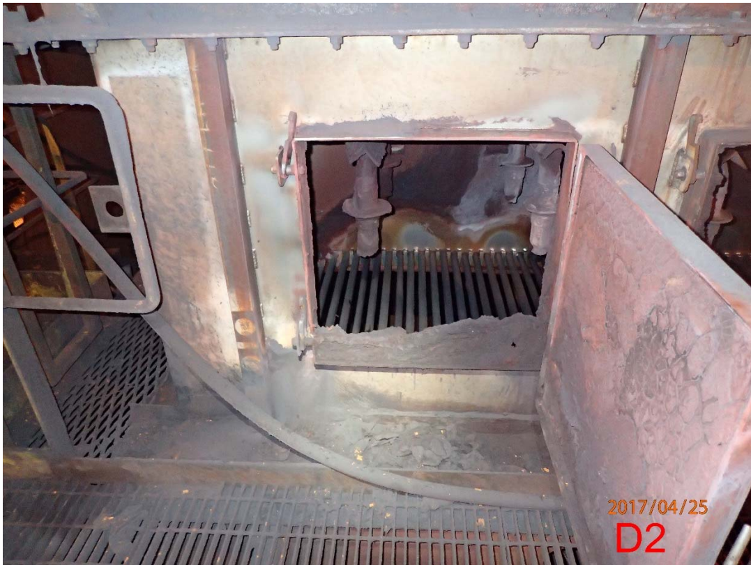
Photo 100 Scrubber D Mid-body (7)
