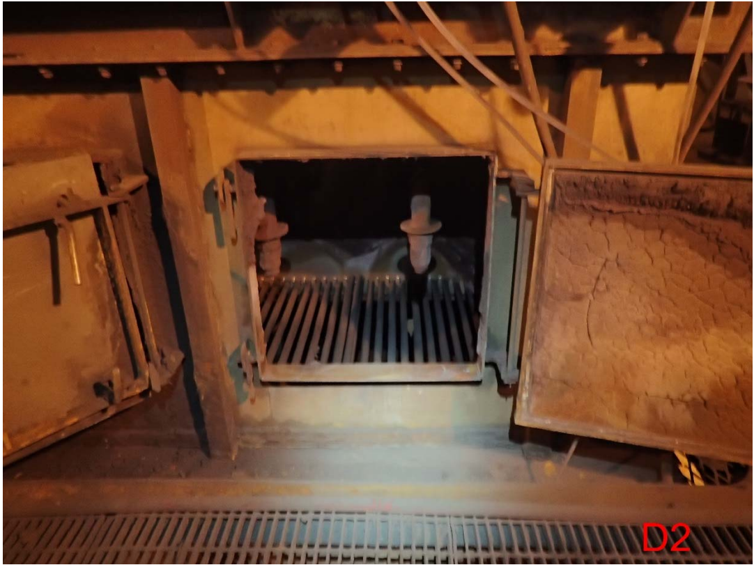
Photo 96 Scrubber D Mid-body (3)
