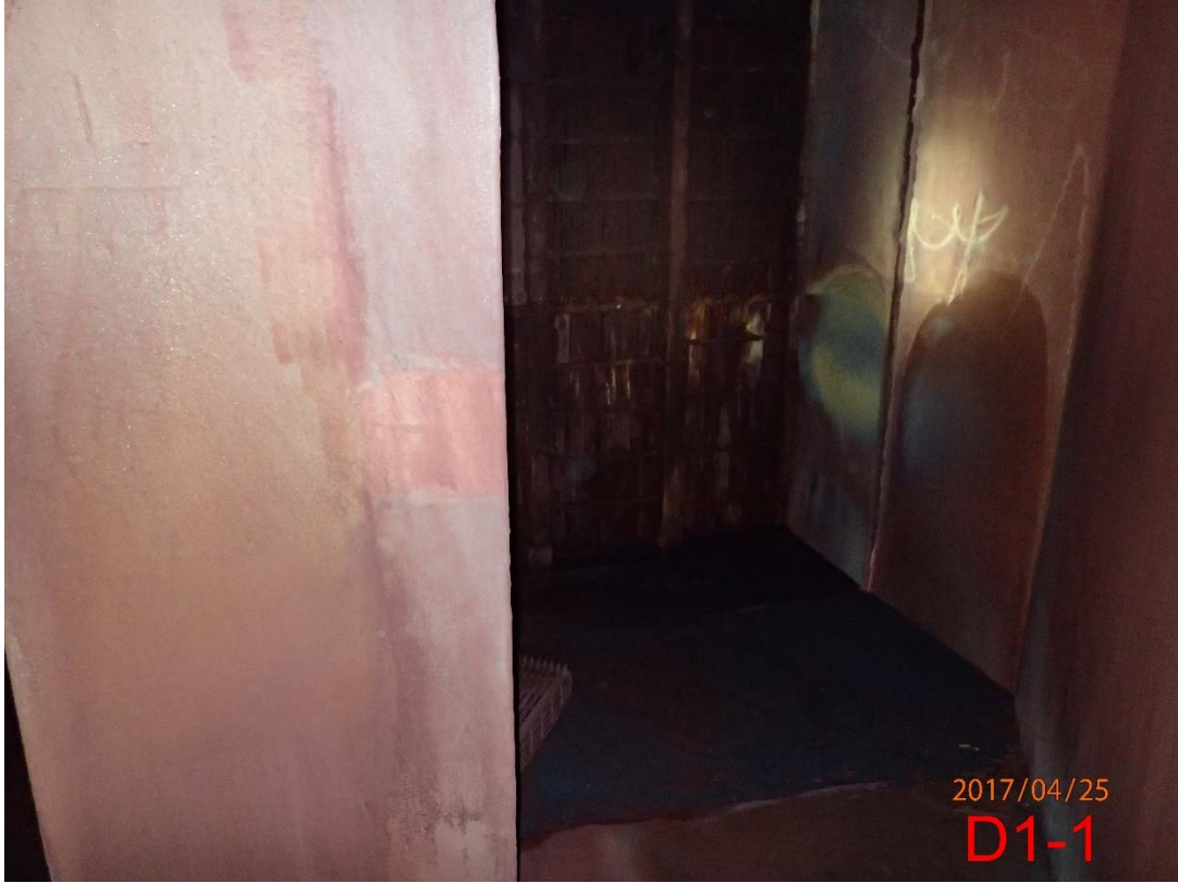
Photo 87 Base of Stack D (7)
