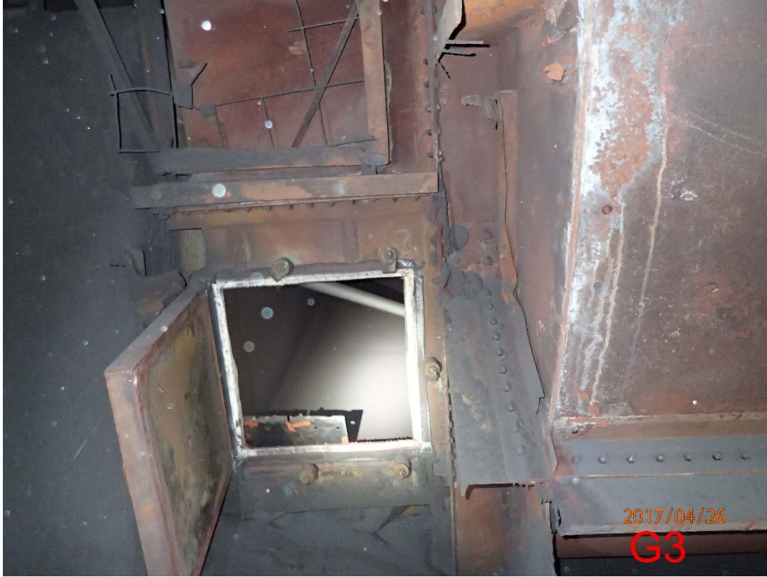
Photo 117 Windbox Inlet Side (1)
