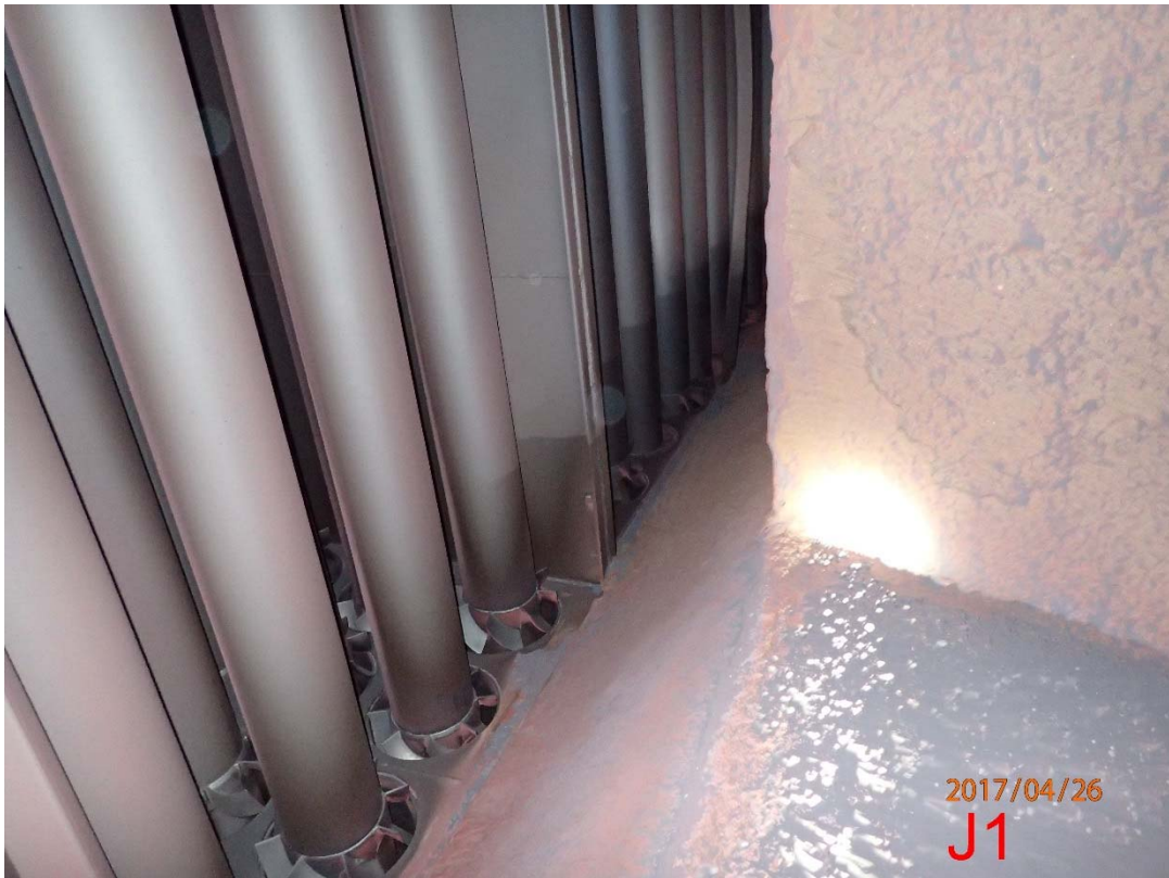
Photo 160 Ducting off Process Gas Header (7)
