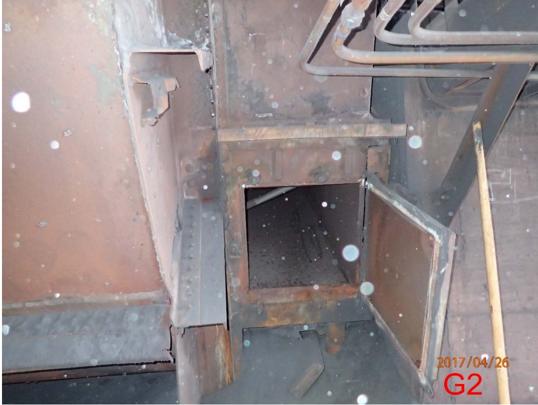
Photo 115 Windbox Outlet Side (1)
