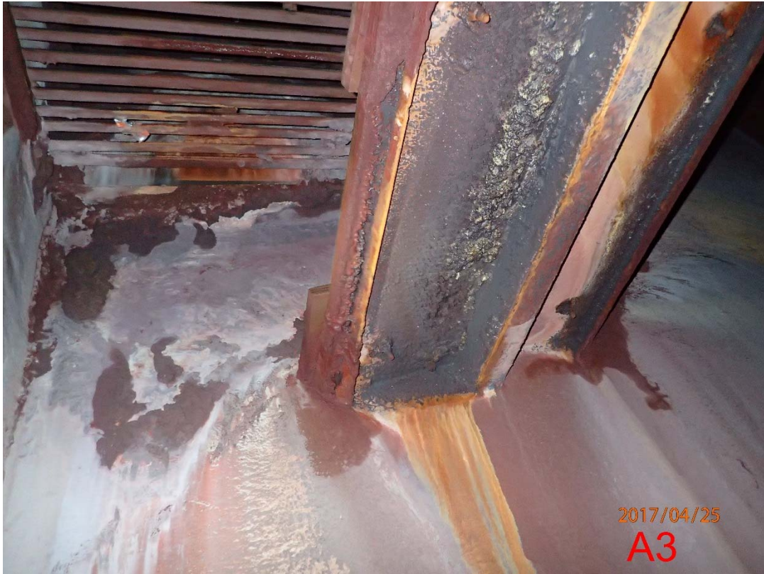
Photo 22 Scrubber A Lower-body (3)
