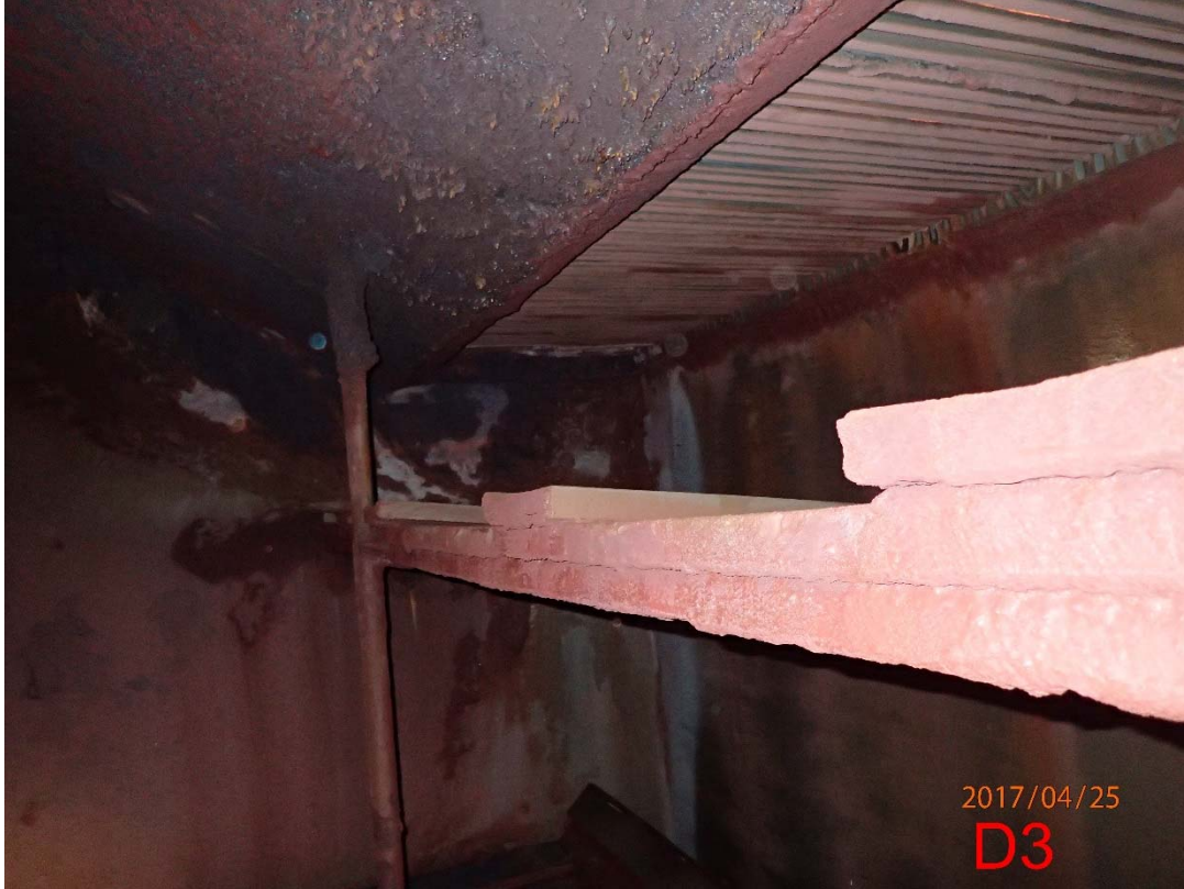
Photo 109 Scrubber D Lower-body (6)
