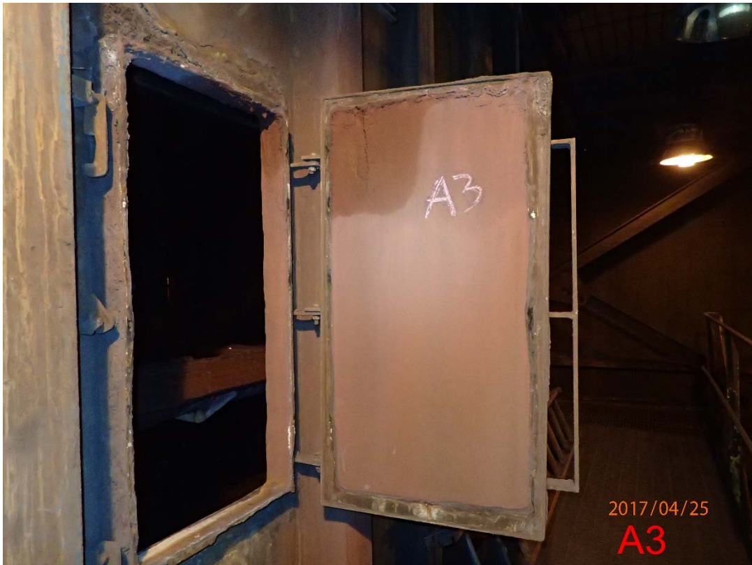
Photo 20 Scrubber A Lower-body (1)
