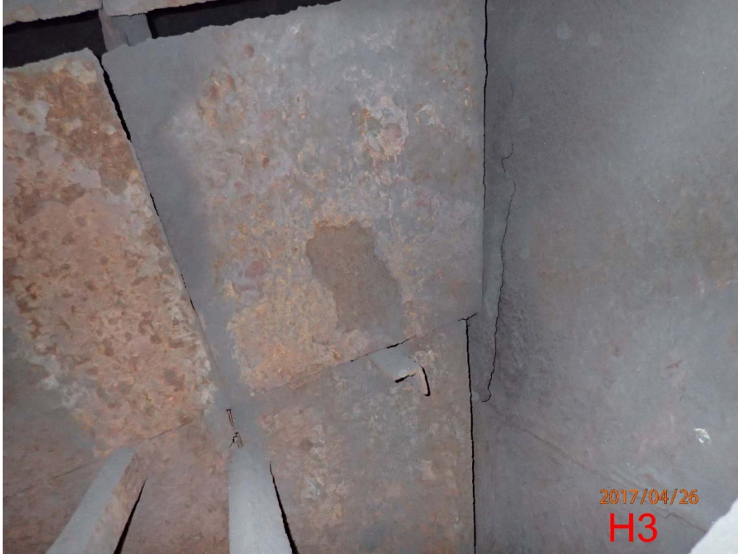
Photo 141 Multiclone Cones at Second Level (14)
