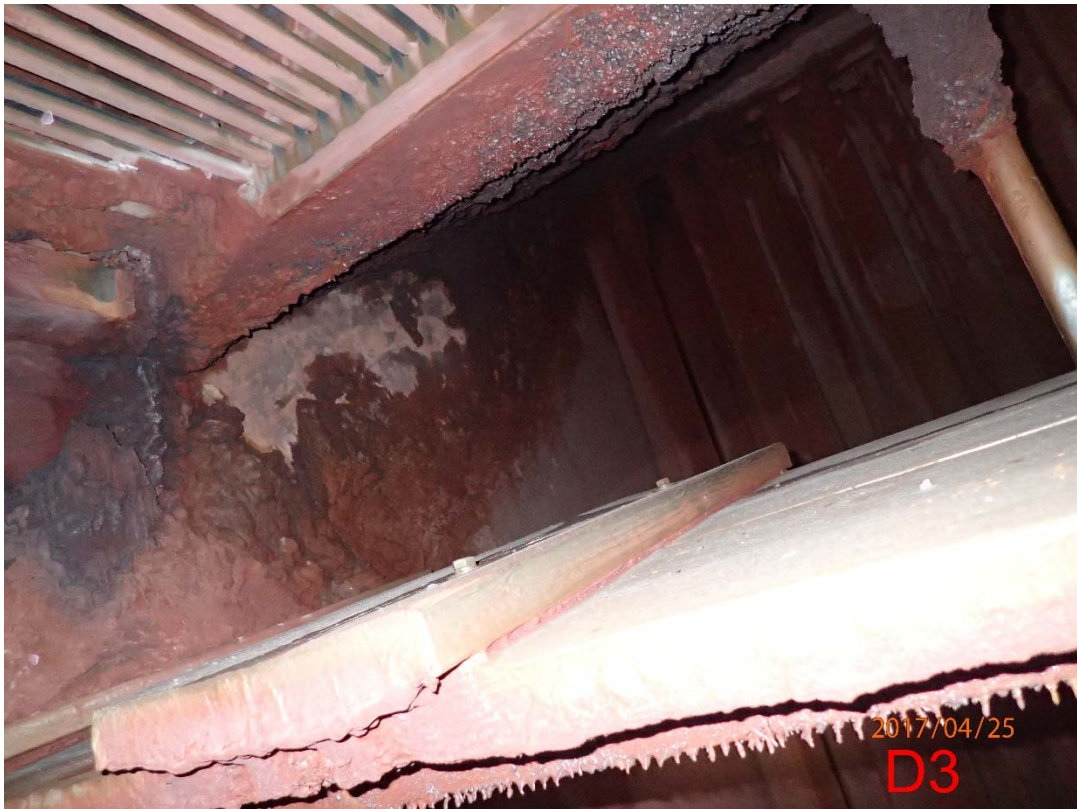
Photo 108 Scrubber D Lower-body (5)
