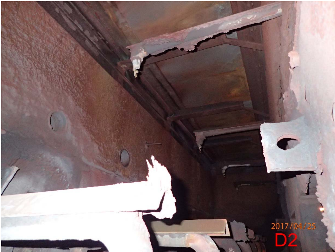
Photo 102 Scrubber D Mid-body (9)
