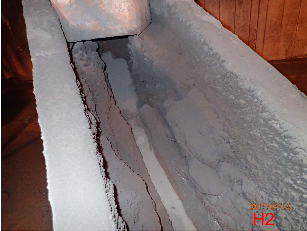
Photo 127 Multiclone Cones Discharge at Ground Level (8)
