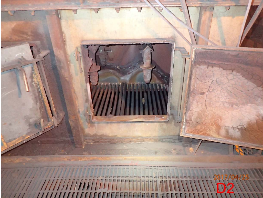
Photo 97 Scrubber D Mid-body (4)
