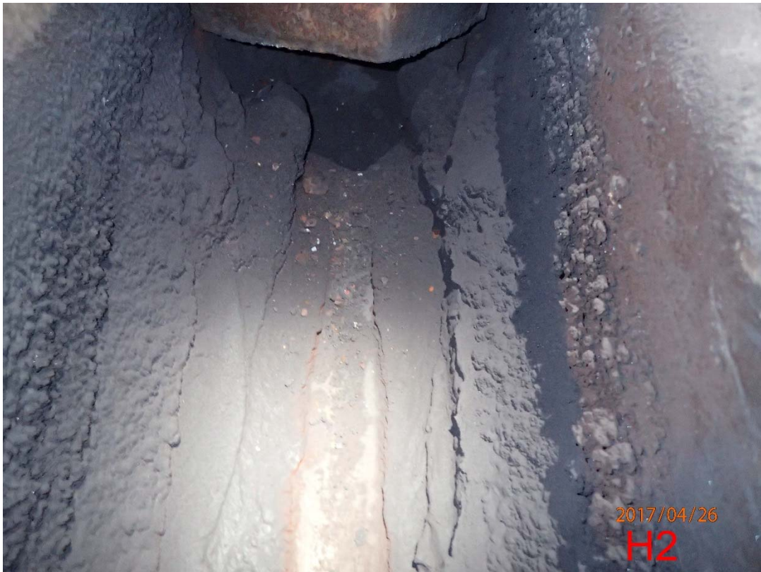
Photo 126 Multiclone Cones Discharge at Ground Level (7)
