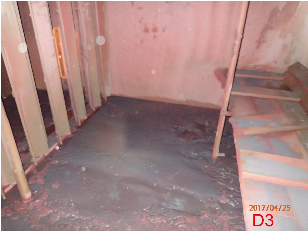
Photo 106 Scrubber D Lower-body (3)
