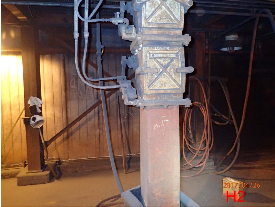
Photo 121 Multiclone Cones Discharge at Ground Level (2)
