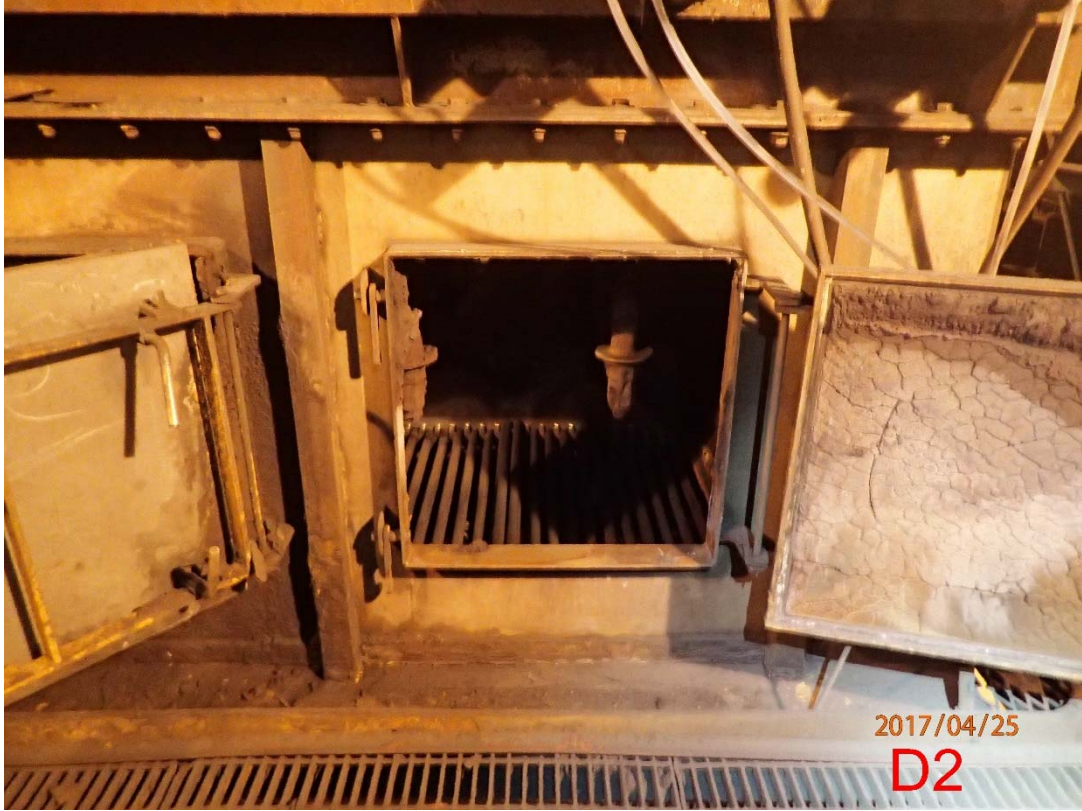
Photo 95 Scrubber D Mid-body (2)
