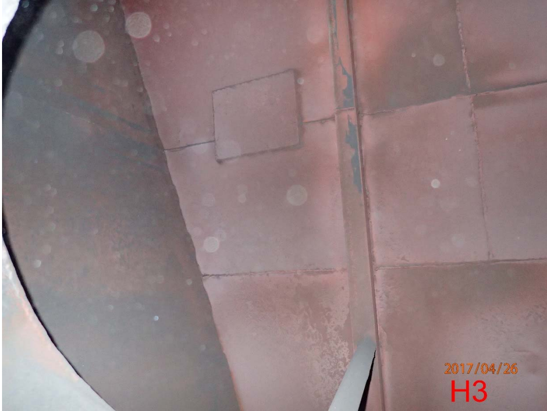
Photo 137 Multiclone Cones at Second Level (10)
