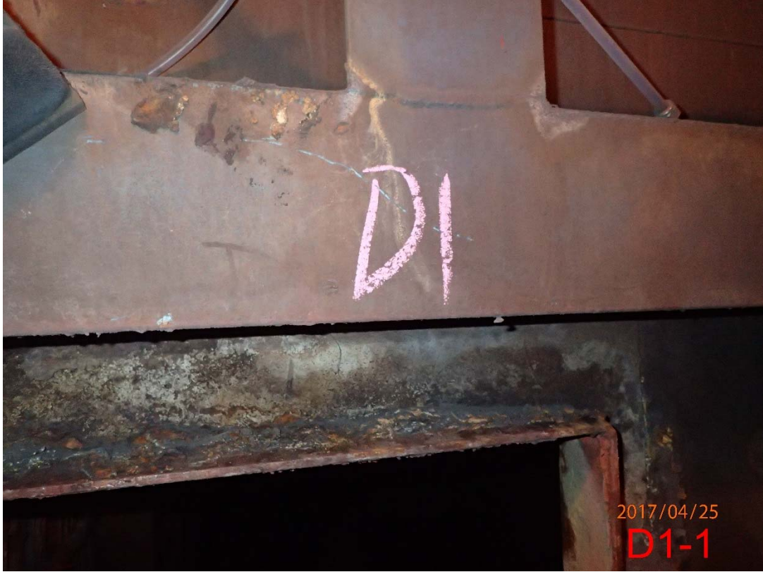
Photo 81 Base of Stack D (1)
