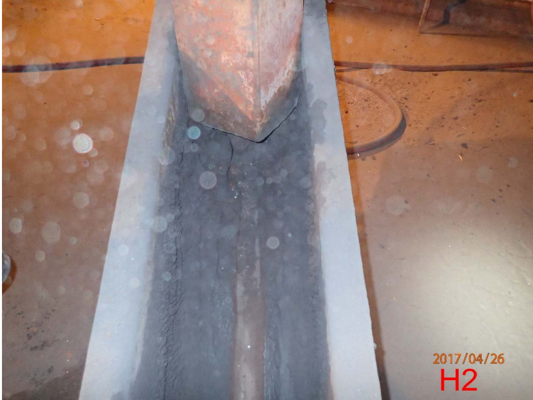
Photo 125 Multiclone Cones Discharge at Ground Level (6)
