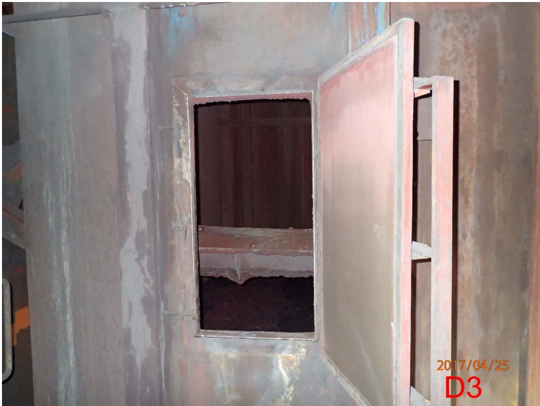
Photo 104 Scrubber D Lower-body (1)
