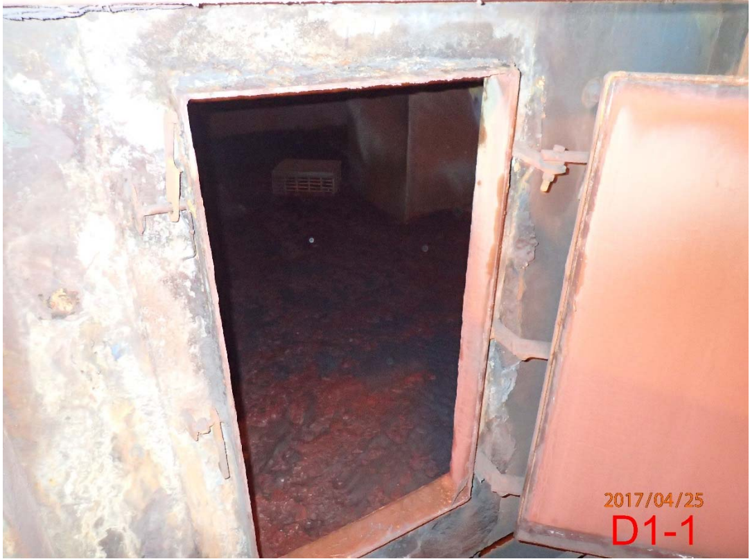
Photo 82 Base of Stack D (2)
