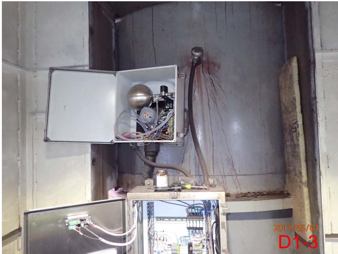
Photo 92 Stack D CEMS Probe (1)
