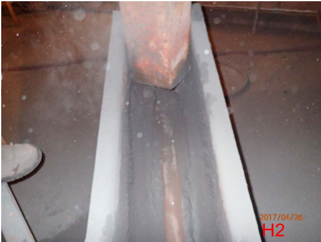
Photo 124 Multiclone Cones Discharge at Ground Level (5)
