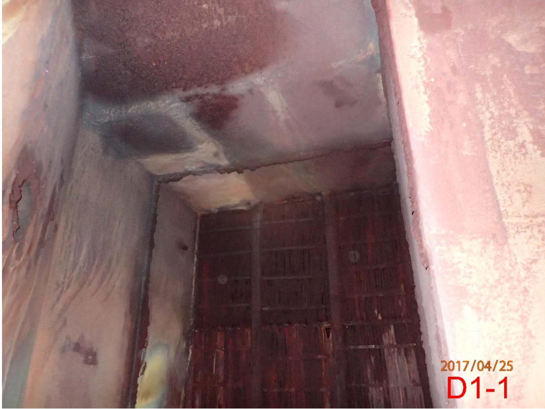
Photo 85 Base of Stack D (5)
