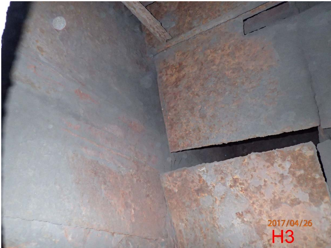
Photo 140 Multiclone Cones at Second Level (13)
