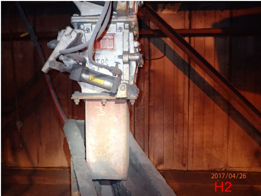
Photo 122 Multiclone Cones Discharge at Ground Level (3)
