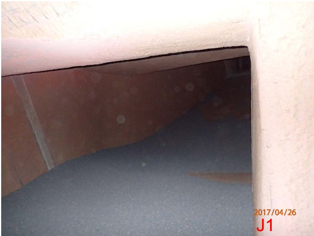
Photo 158 Ducting off Process Gas Header (5)
