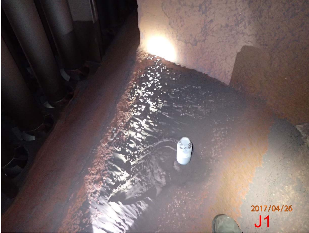
Photo 163 Ducting off Process Gas Header (10)
