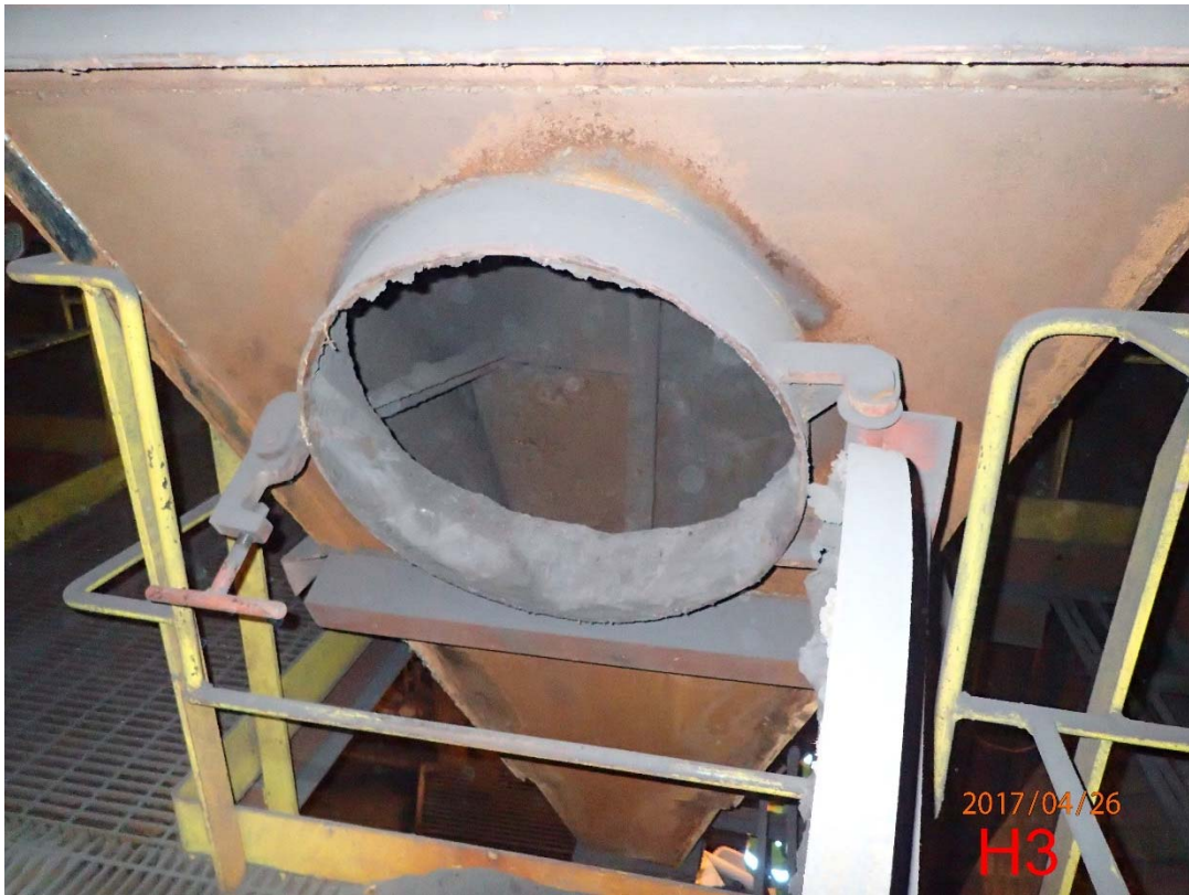
Photo 128 Multiclone Cones at Second Level (1)
