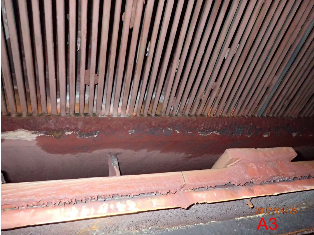
Photo 25 Scrubber A Lower-body (6)
