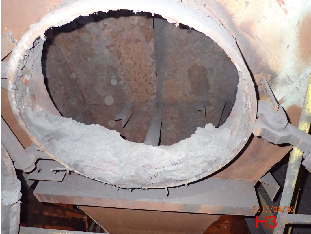
Photo 139 Multiclone Cones at Second Level (12)
