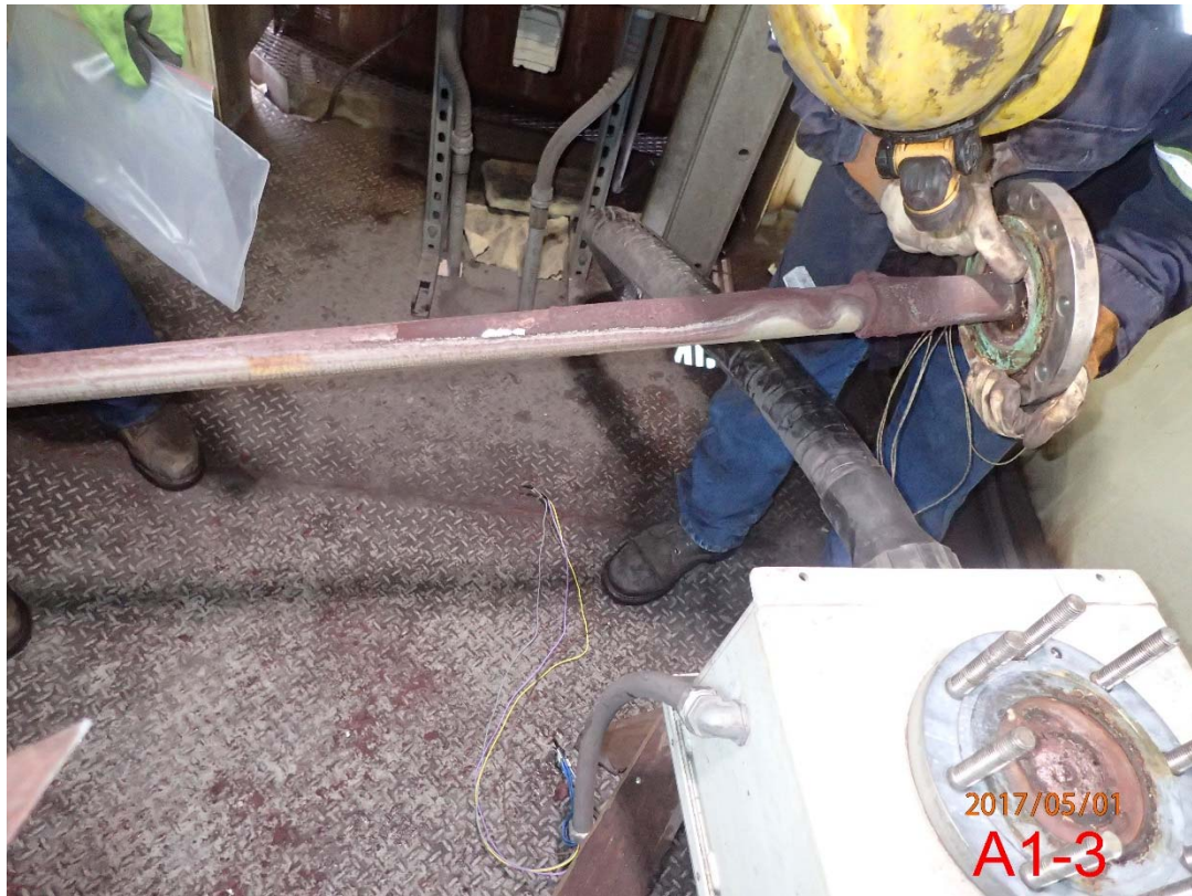
Photo 10 Stack A CEMS Probe (1)
