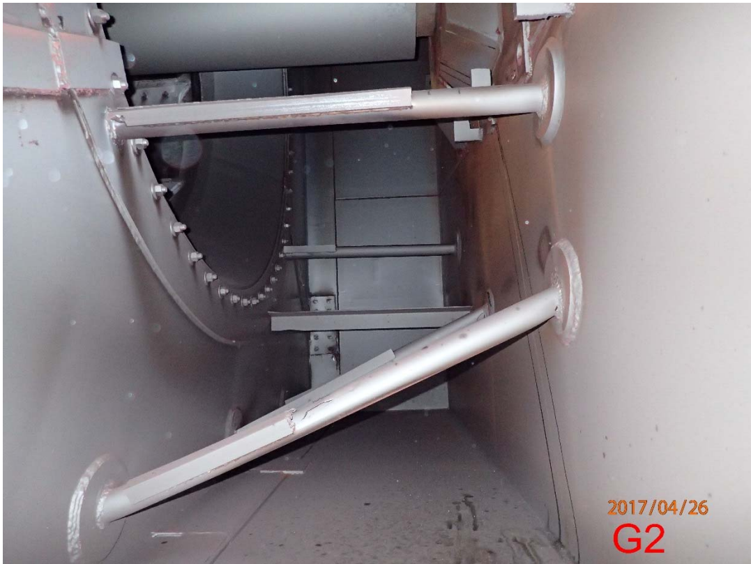
Photo 116 Windbox Outlet Side (2)
