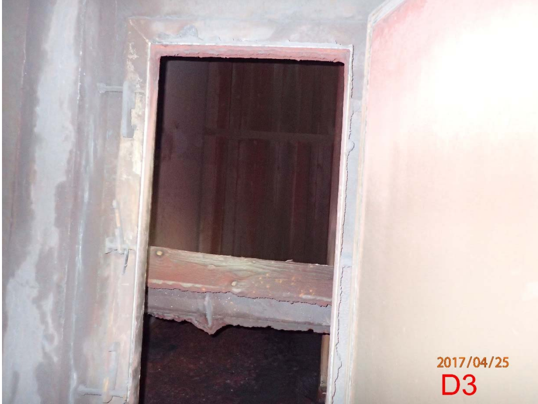
Photo 105 Scrubber D Lower-body (2)
