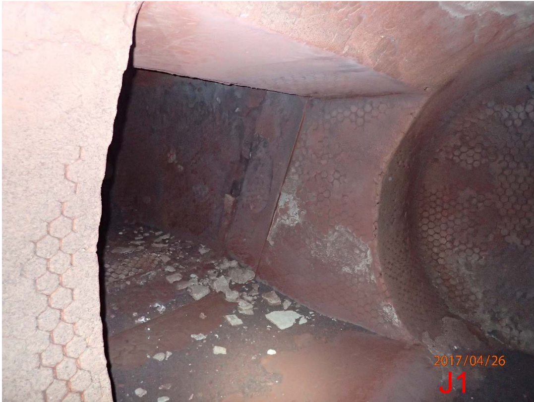
Photo 155 Ducting off Process Gas Header (2)
