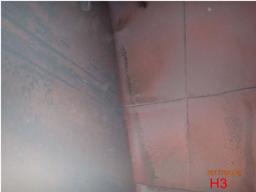
Photo 144 Multiclone Cones at Second Level (17)
