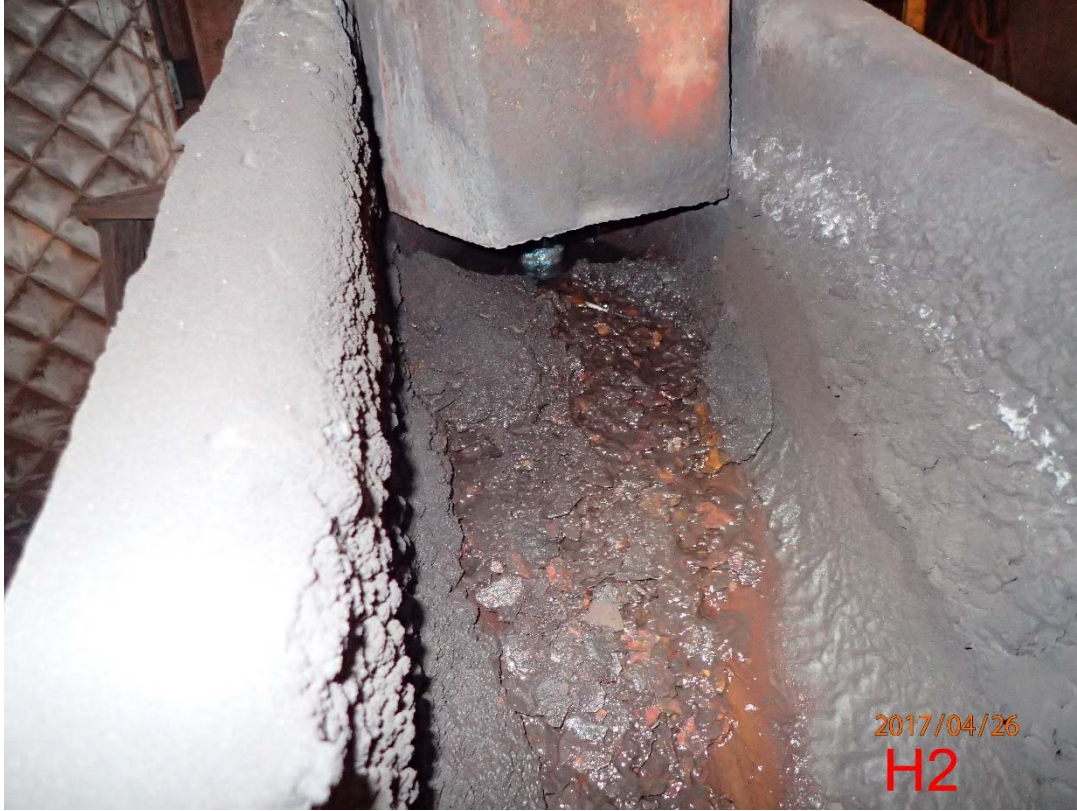
Photo 123 Multiclone Cones Discharge at Ground Level (4)
