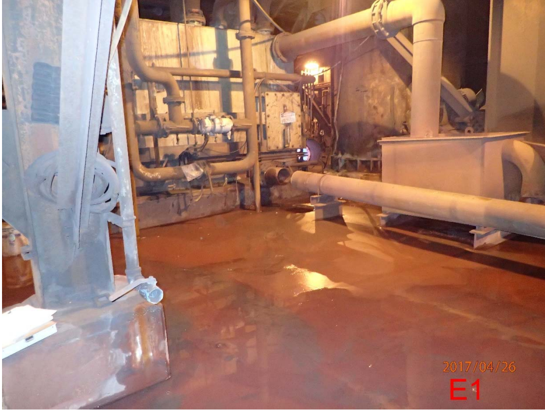
Photo 111 Scrubber Recirculating Tank
