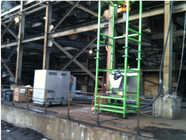
Figure 2: Bulk Bag Unloader location and setup
