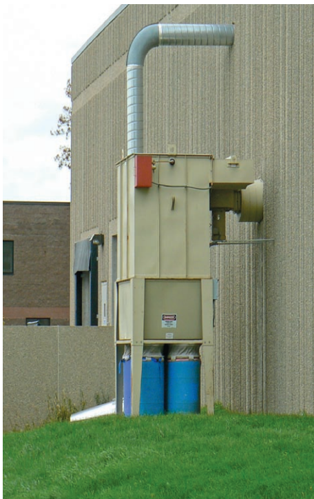
Pollution control equipment like this dust collector needs to be sheltered to qualify for the No Exposure Exclusion.
