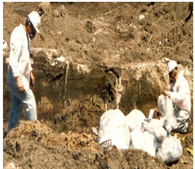
Licensed contractors removing asbestos waste material from a site near the University of Minnesota in Minneapolis.
