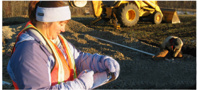
A Becker County supervisor oversees the installation of an SSTS at a site a few miles south of Detroit Lakes.
