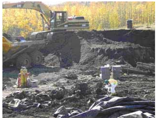
MPCA contractors excavated and disposed of more than 9,500 barrels (filled mostly with leaded gear lube) at the former Reserve Mining Superfund site on what is now North Shore Mining property in Silver Bay.
